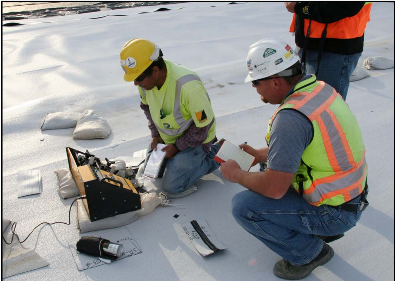
Workers test the welds on the primary high-density polyethylene layer in super cell 9 at the Environmental Restoration Disposal Facility.
