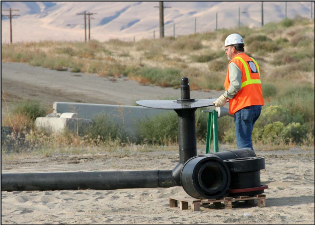
Work to install piping for leachate holding tank No. 4 began at the Environmental Restoration Disposal Facility. The new holding tank will have a capacity of 420,000 gallons.
