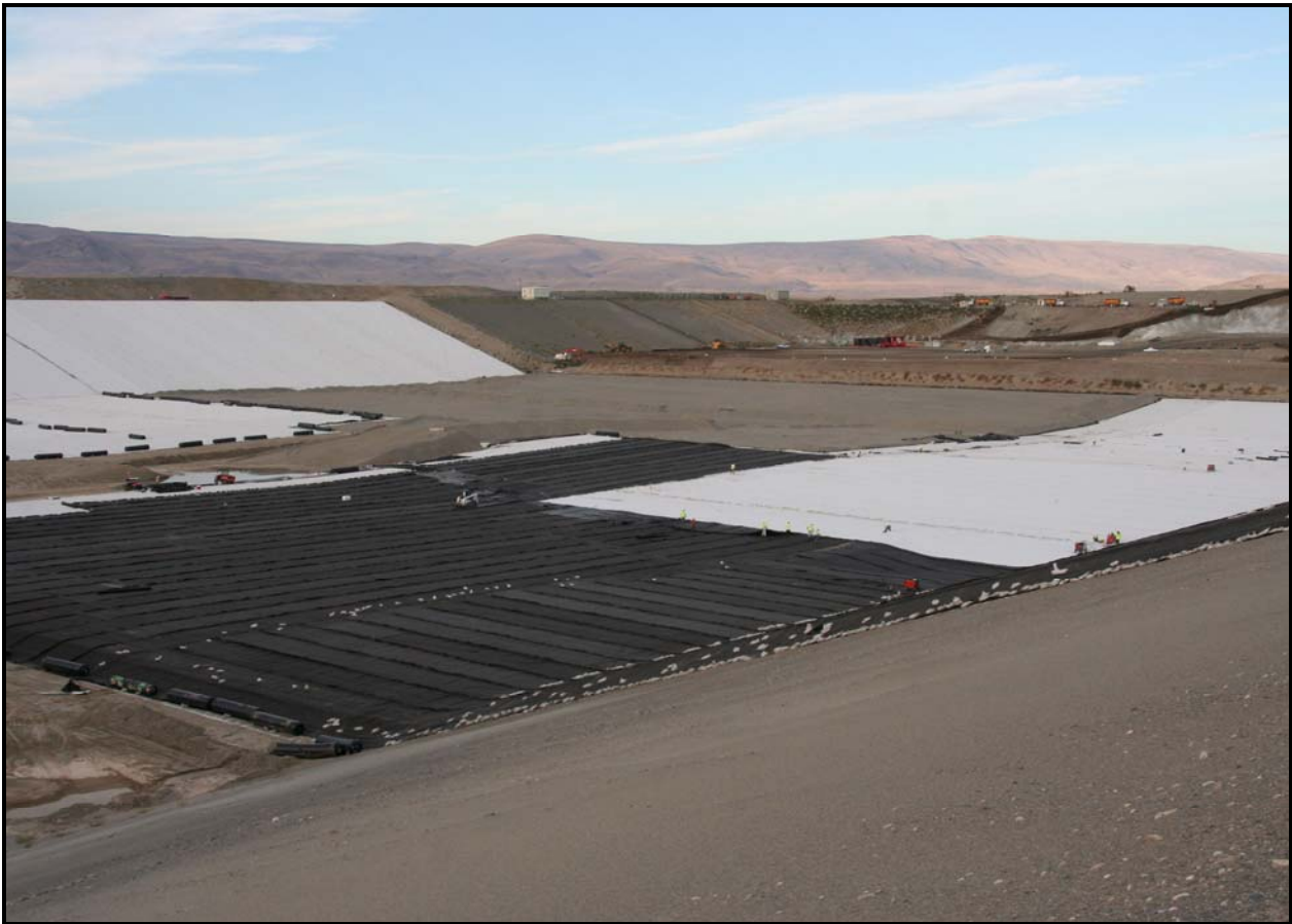
A view from the northeast corner of super cell 10 shows liner construction progress at the Environmental Restoration Disposal Facility.
