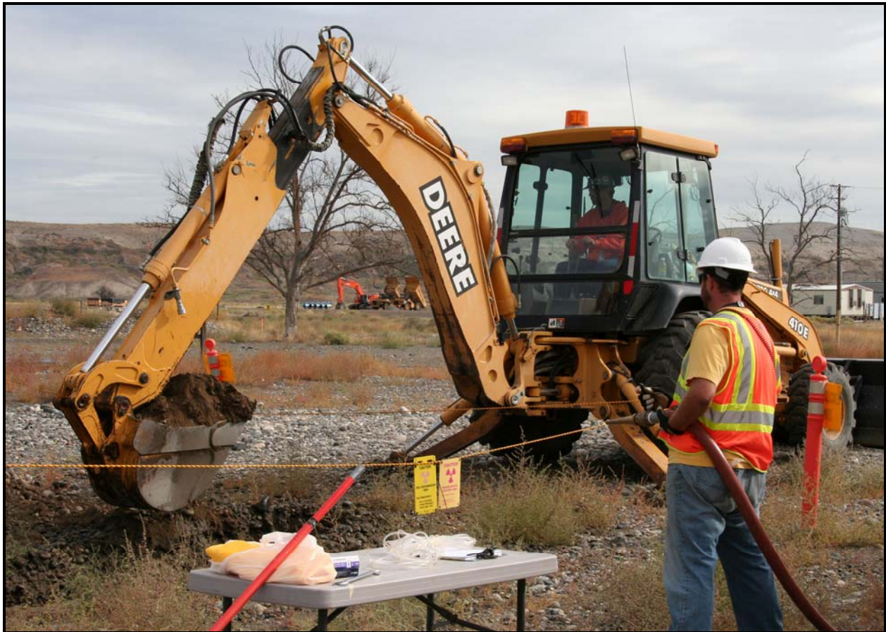
Workers excavate a test pit at site 100-F-26:4. The site contains a section of process sewer pipeline.
