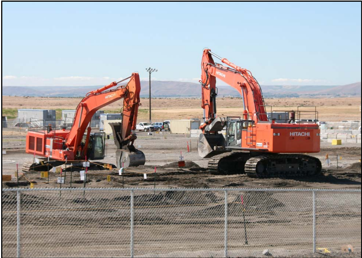
Waste trench excavation continues at the 618-10 Burial Ground. Trench excavation work is about 20% complete. (Photo 7)
