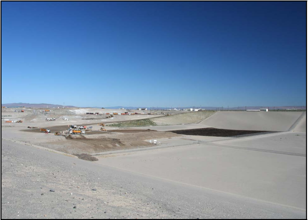
A view from the southeast corner of the Environmental Restoration Disposal Facility shows disposal activities in super cell 9. (Photo 1)
