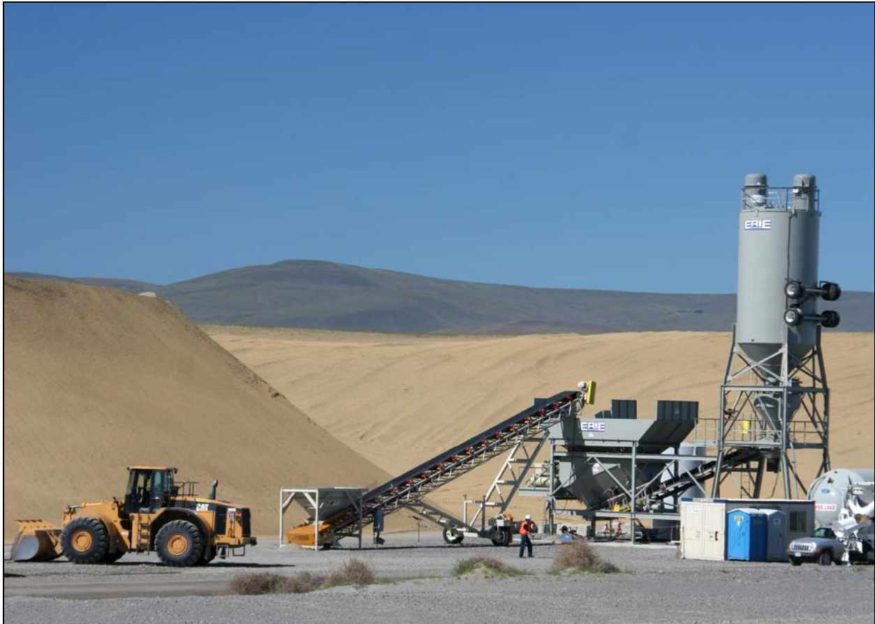
The new batch plant at the Environmental Restoration Disposal Facility has been tested. The plant's operating procedures are being finalized before the plant is placed into service. (Photo 6)
