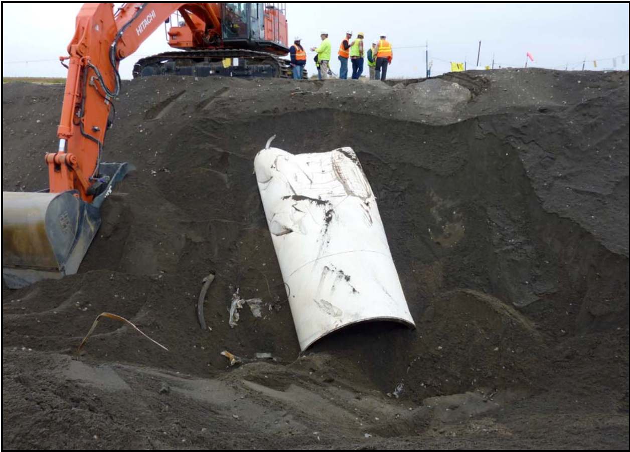
The steel tank found at the 618-10 Burial Ground contained a ladder. (Photo 7)
