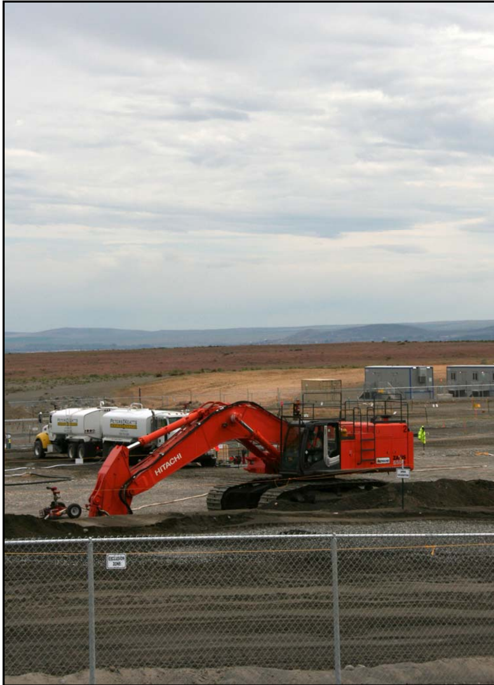
Washington Closure Hanford continues excavation of the waste trenches at the 618-10 Burial Ground. (Photo 6)
