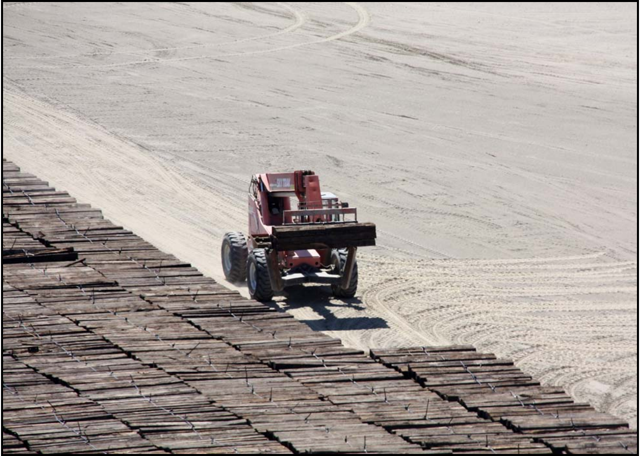
The Waste Operations team continues to place railroad ties in super cell 9. Approximately 65,000 ties will cover about half of the super cell floor. The Hanford Site had more than 150 miles of railroad track, only a fraction of which is still in use. (Photo 2)
