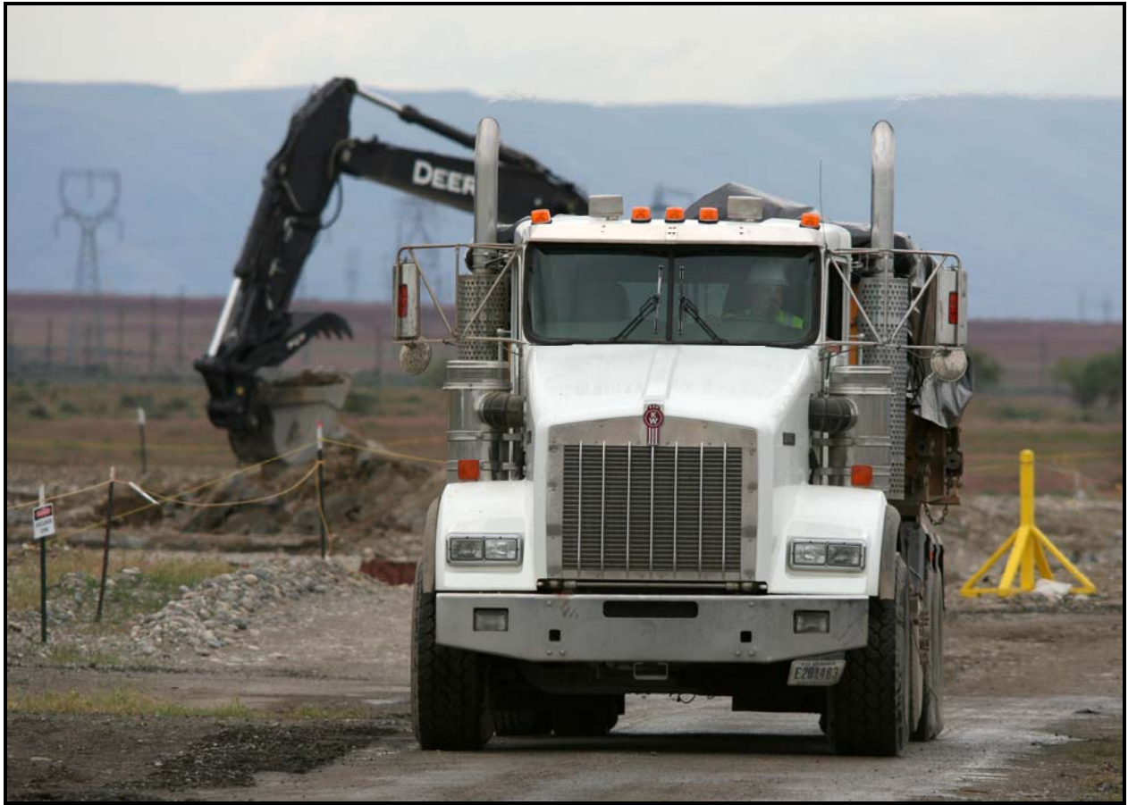
Concrete and soil from 100-F-57 is loaded out and transported to the Environmental Restoration Disposal Facility. (Photo 10)
