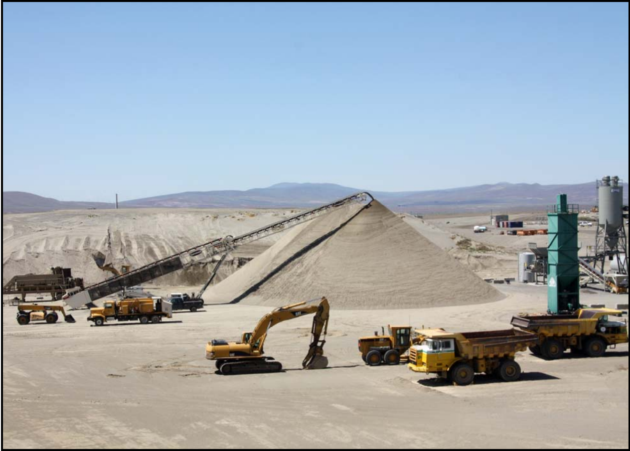
The new screener for the batch plant is operational at the Environmental Restoration Disposal Facility. The batch plant, which will manufacture concrete for disposal, is expected to be in service this month. (Photo 5)
