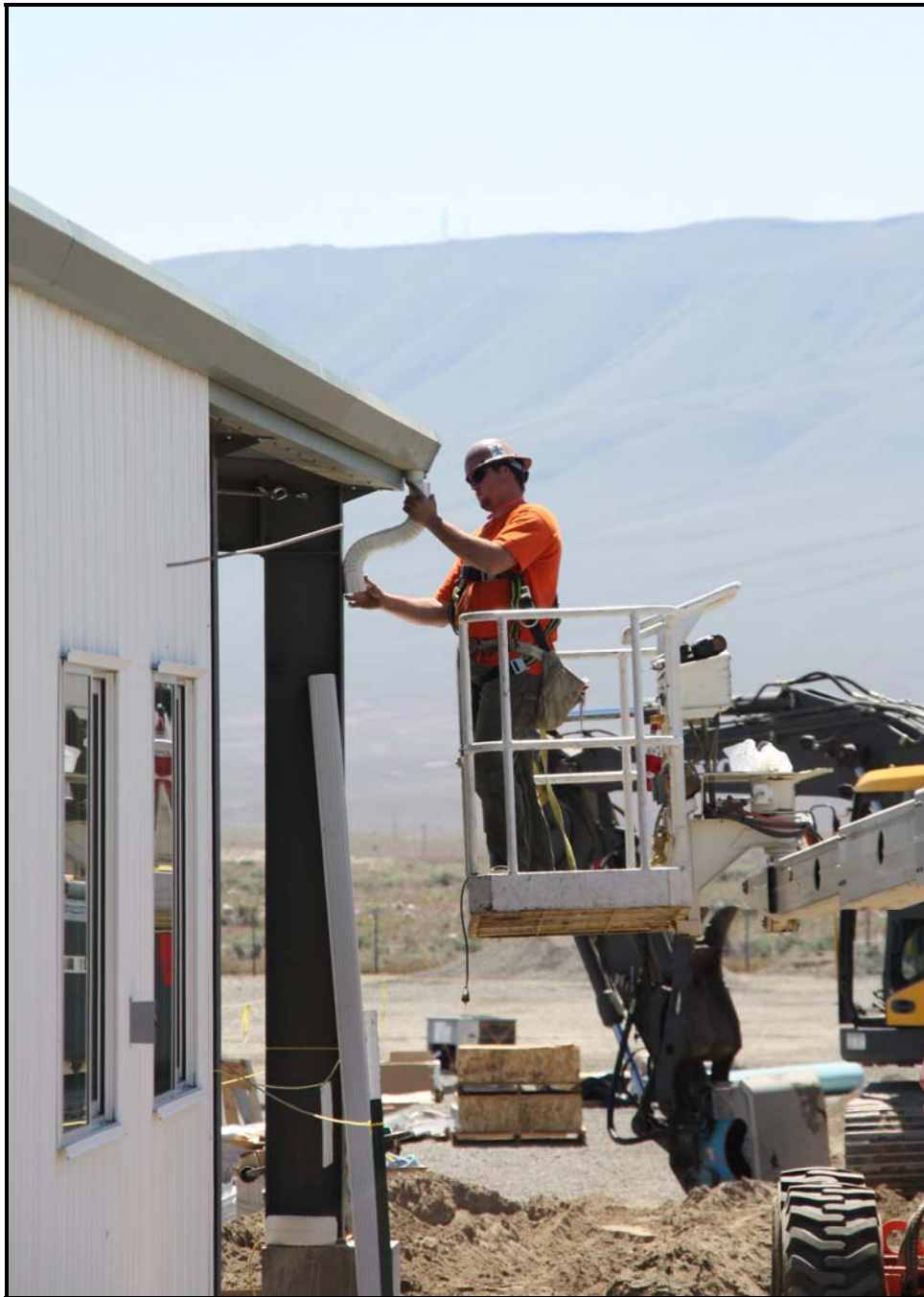
An employee with Washington Closure Hanford subcontractor ELRFowler installs gutters on the west addition of the transportation maintenance facility. (Photo 3)
