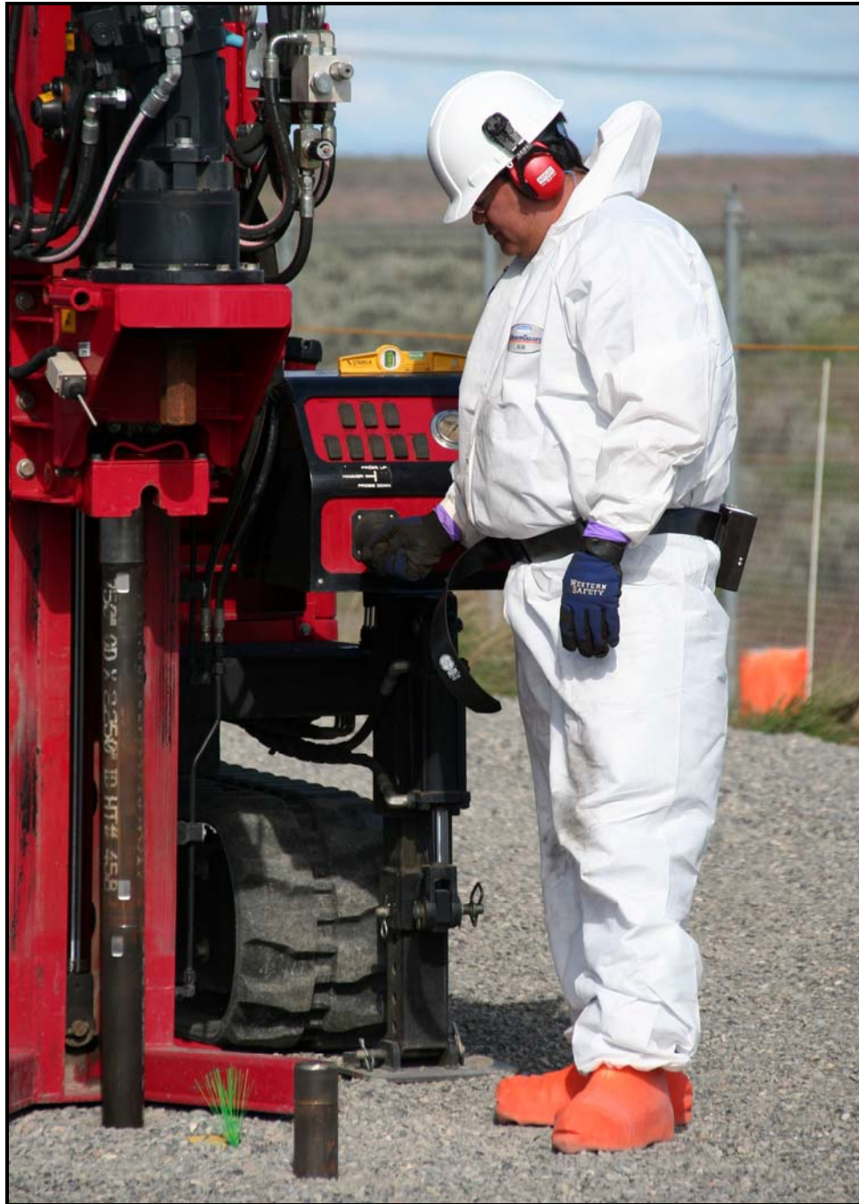
An employee with Washington Closure Hanford subcontractor North Wind installs one of 100 cone penetrometers at the 618-11 Burial Ground. (Photo 8)
