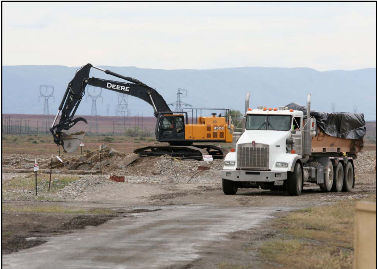
Washington Closure Hanford subcontractor Ojeda Business Ventures continues to demolish and load out concrete and soil from 100-F-57. (Photo 9)
