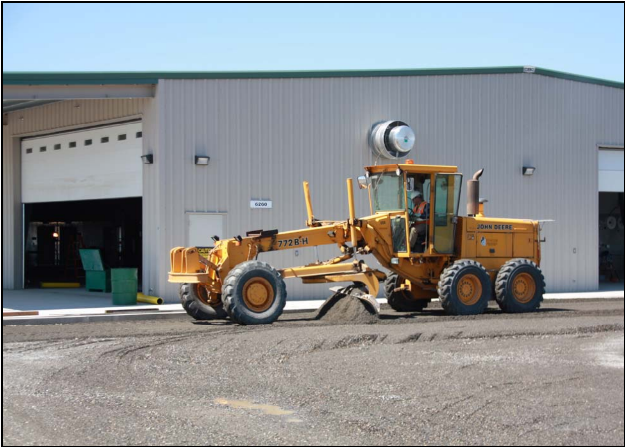
An ELRFowler employee spreads gravel for the parking area on the east side of ERDF's new container maintenance facility. (Photo 4)
