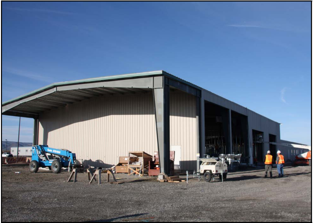
ELRFowler completed installation of the siding and roofing at ERDF's equipment maintenance facility/operations center. (Photo 4)
