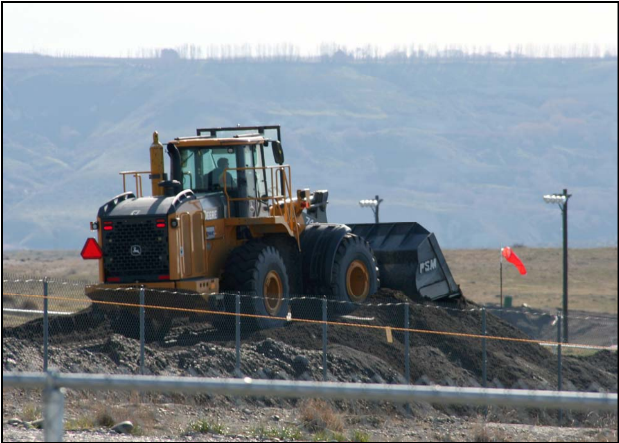
A front-end loader moves soil during surge trench excavation activities at the 618-10 Burial Ground. (Photo 7)
