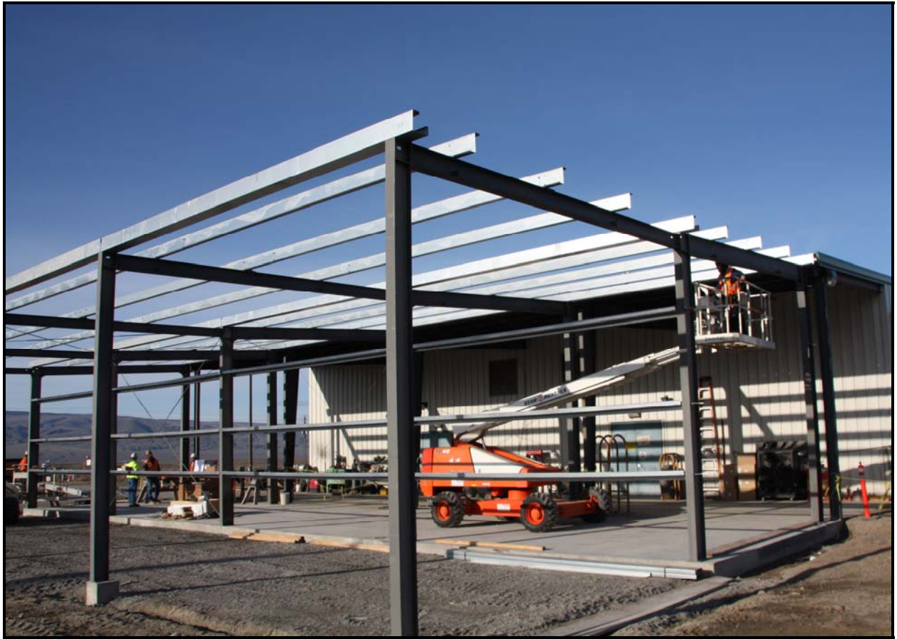
Two new truck bays are being added to ERDF's transportation maintenance facility. The new facility will help ERDF personnel safely and efficiently handle increased waste volumes. (Photo 3)
