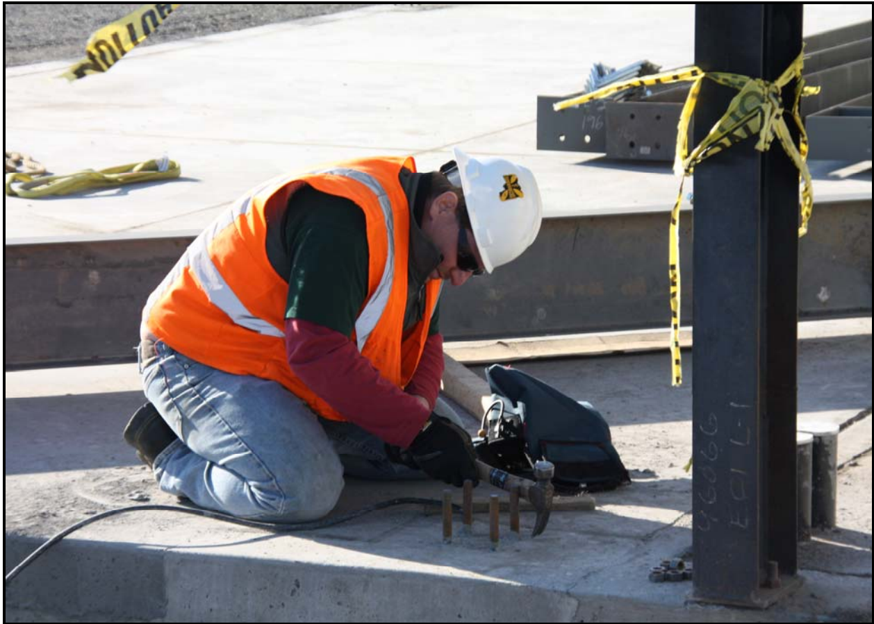
An employee with Washington Closure Hanford subcontractor ELRFowler prepares to stand a piece of structural steel at the east addition of ERDF's transportation maintenance facility. (Photo 1)
