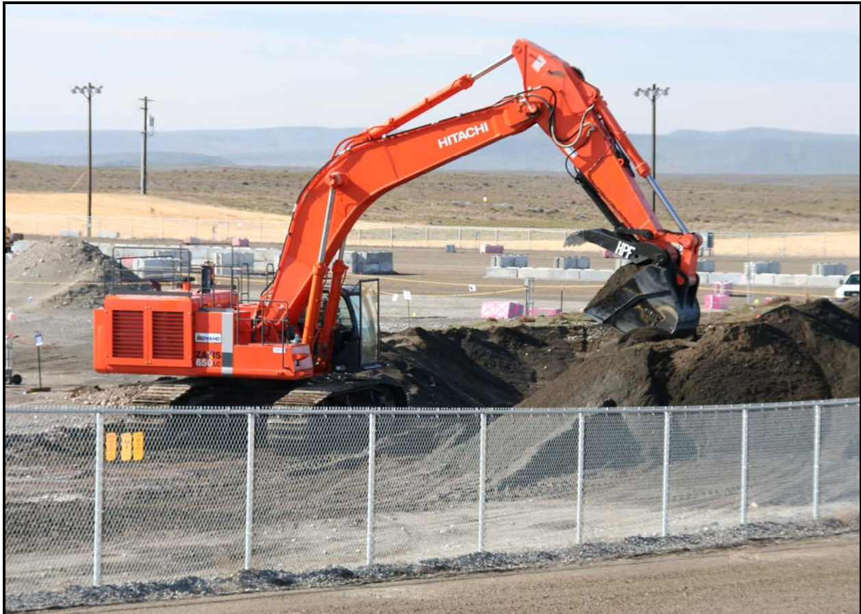
Washington Closure Hanford begins excavating surge trenches at the 618-10 Burial Ground. (Photo 6)
