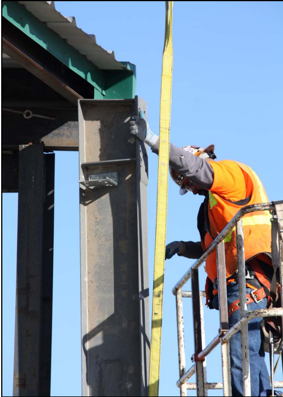
ELRFowler erects structural steel for the east addition of the transportation maintenance facility at ERDF. (Photo 2)
