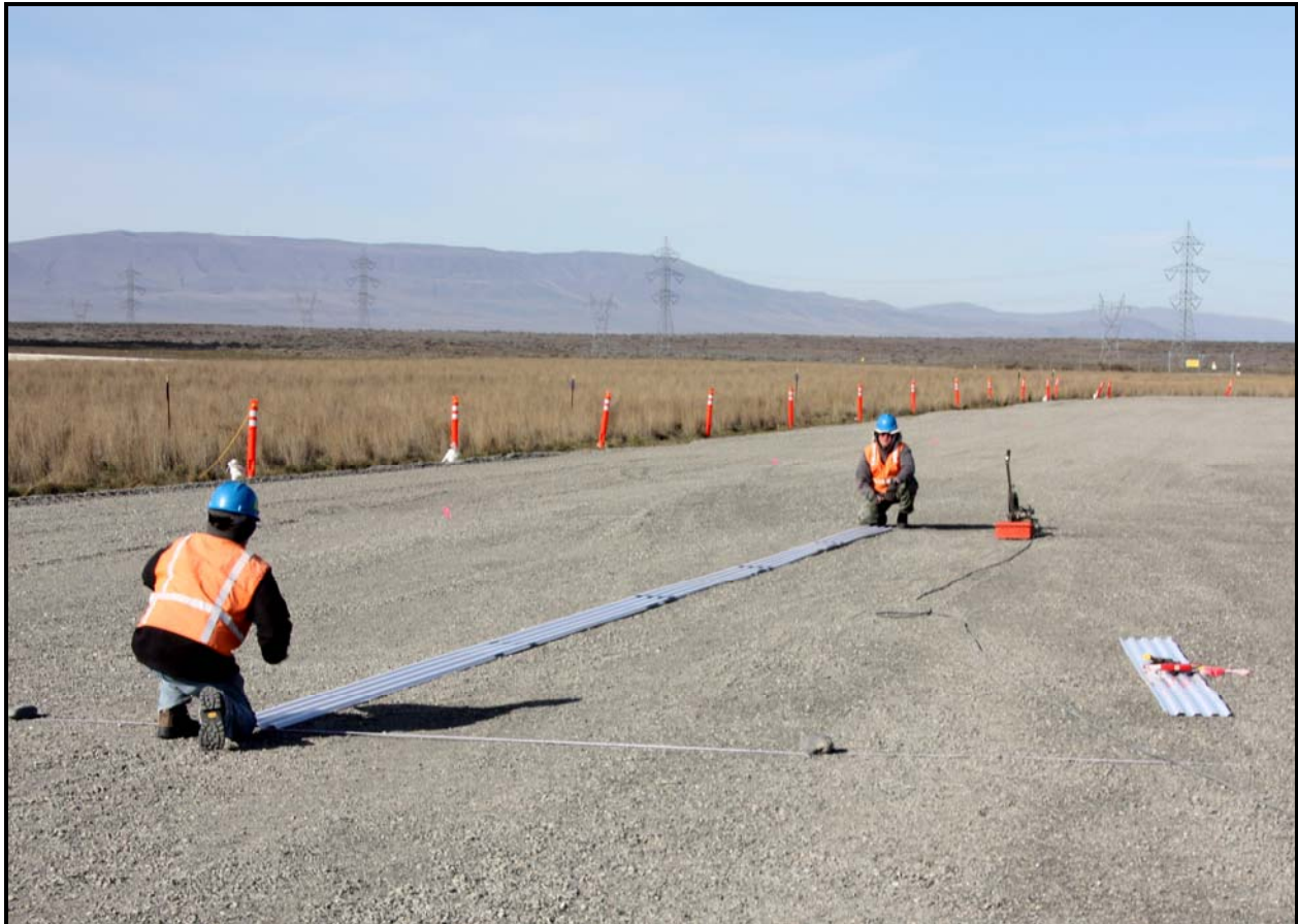
Workers from Washington Closure Hanford subcontractor Sage Earth Science of Idaho Falls, Idaho, prepare for geophysical delineation at the 618-11 Burial Ground. (Photo 8)
