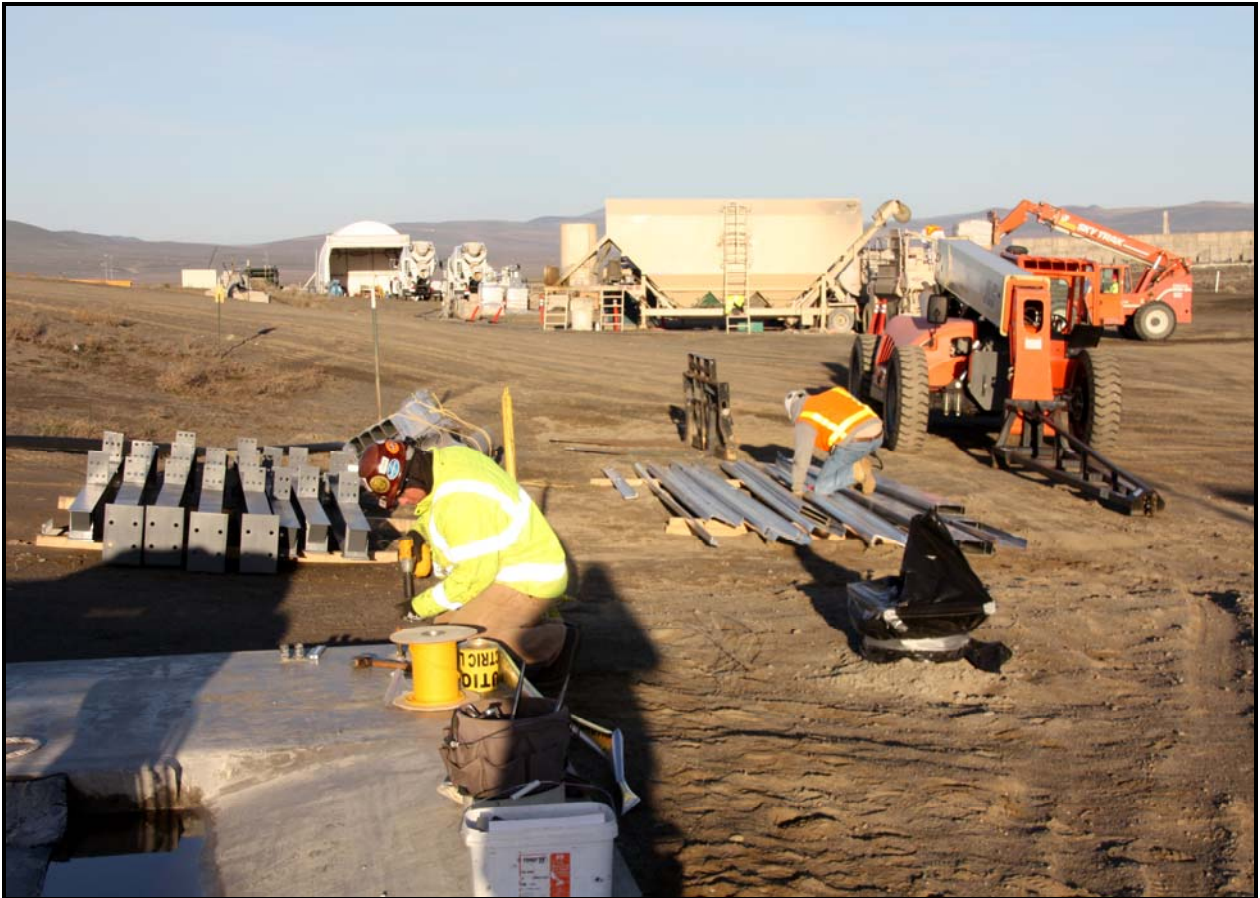
Work is under way to construct the steel structures for crest pad buildings for cells 1 and 2. (Photo 5)
