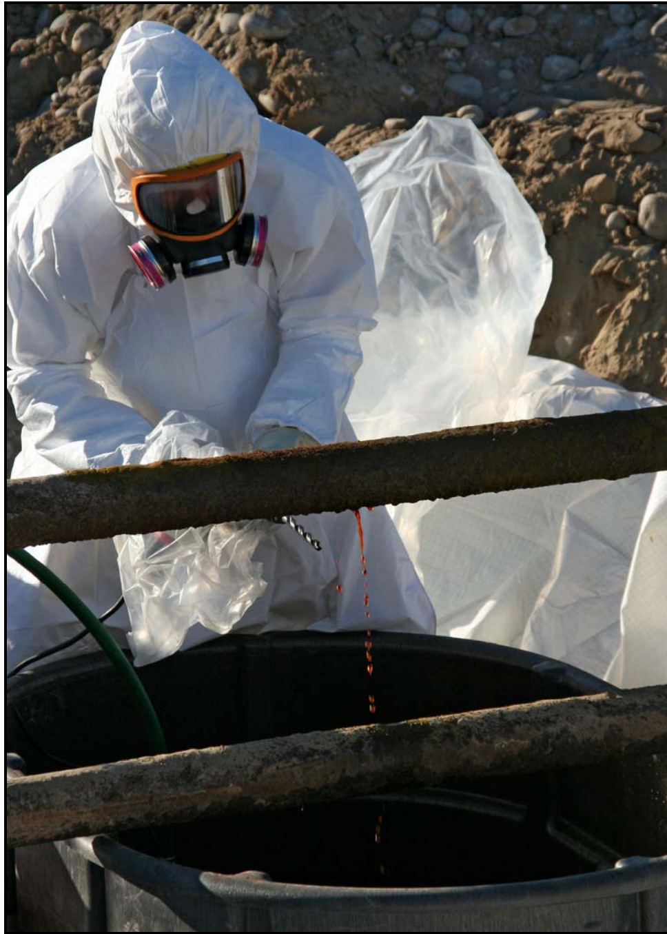
A worker drills a hole to drain liquid from a pipe at 110-F-26:7. (Photo 11)
