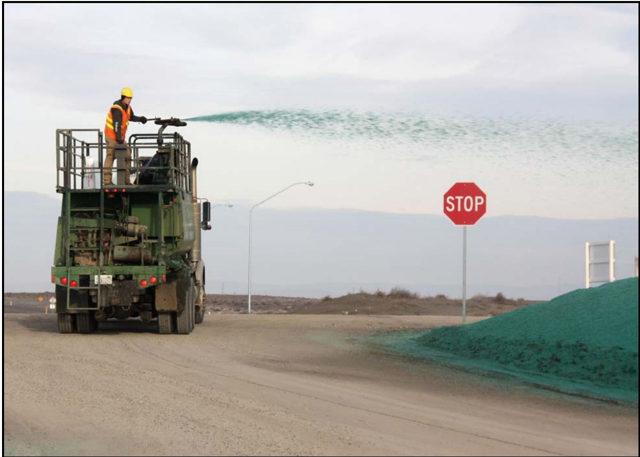
Washington Closure Hanford subcontractor Wildlands spreads hydroseed at the 618-10 Burial Ground. The hydroseed will help with dust suppression and erosion. (Photo 5)
