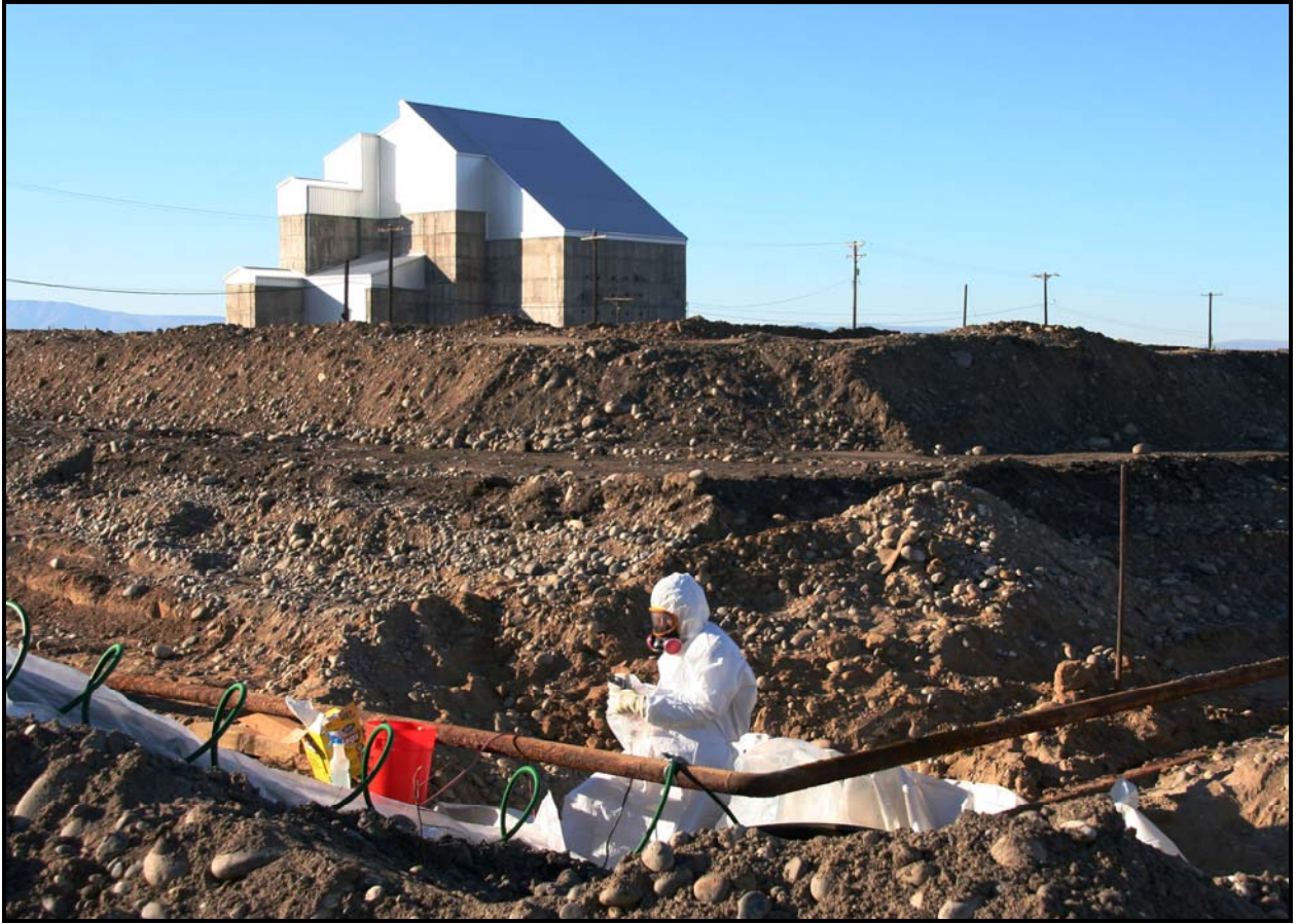
A worker cuts and drains pipe at 100-F-26:7, which contains sodium dichromate and sodium silicate pipelines. (Photo 10)
