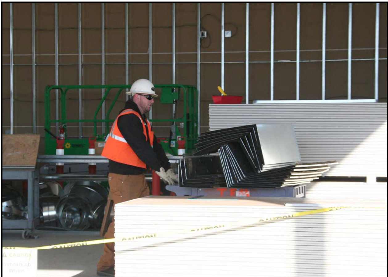
An employee with Washington Closure Hanford subcontractor ELRFowler works to install sheetrock in the new container maintenance facility at ERDF. (Photo 3)
