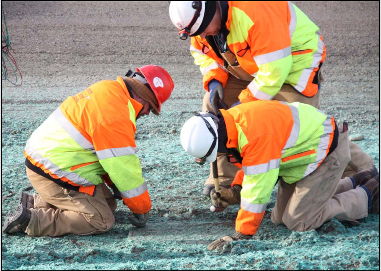
Workers are close to completing installation of the electrical system at the 618-10 Burial Ground. (Photo 7)
