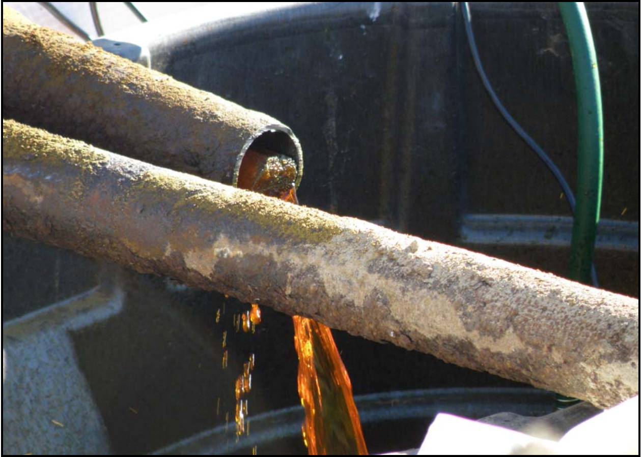
A pipe is cut and liquid drains out at 100-F-26:7. (Photo 12)
