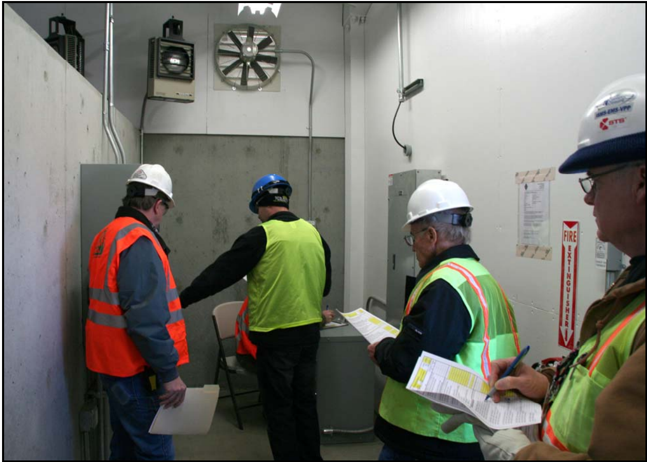
Washington Closure Hanford subcontractor TradeWind Services test the trench pump control panel in crest pad building 10 during final acceptance testing of Leachate Storage Tank No. 4. The testing was conducted with the U.S. Department of Energy and the U.S. Environmental Protection Agency. (Photo 1)
