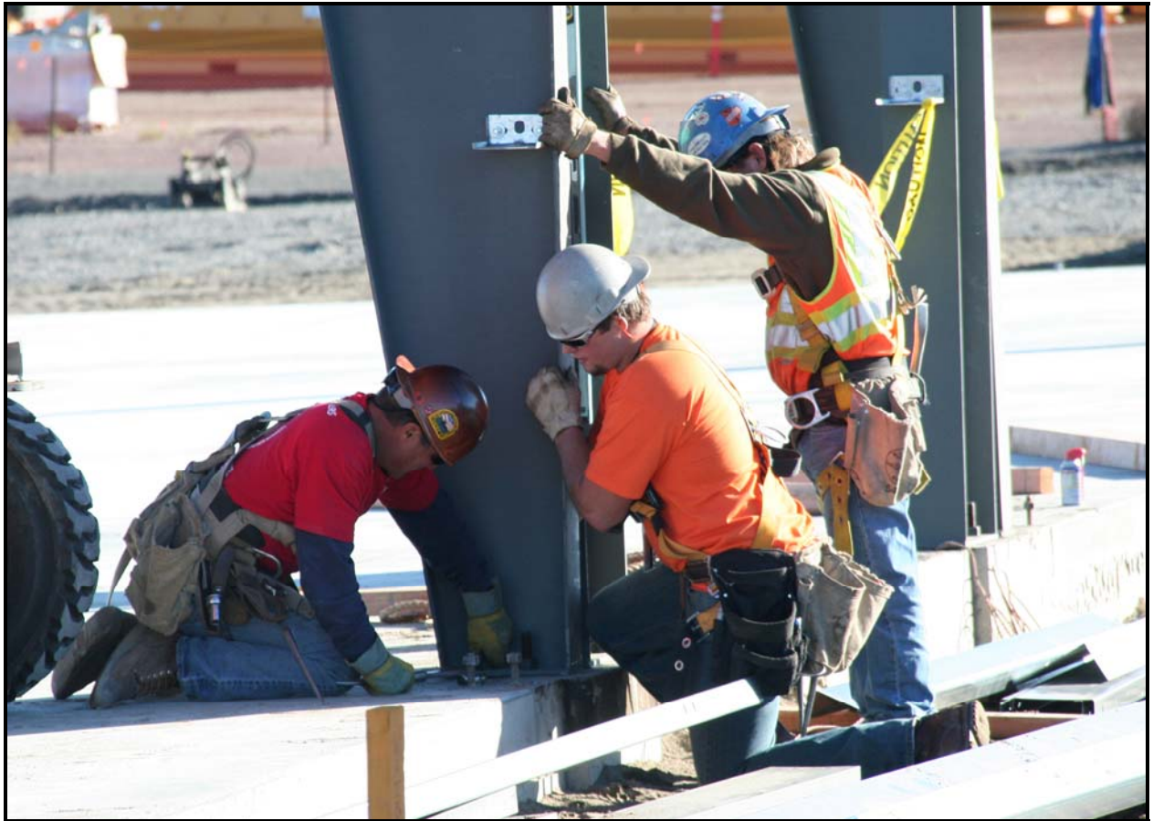
Washington Closure Hanford subcontractor Fowler General Construction begins to erect steel for the container maintenance facility at the Environmental Restoration Disposal Facility. (Photo 4)
