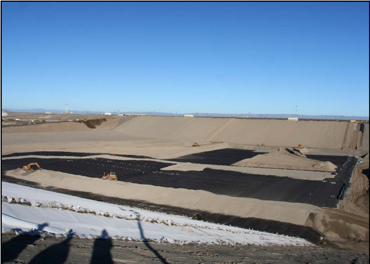
A view from the northwest corner of super cell 9 shows construction progress of both super cells at the Environmental Restoration Disposal Facility. (Photo 1)
