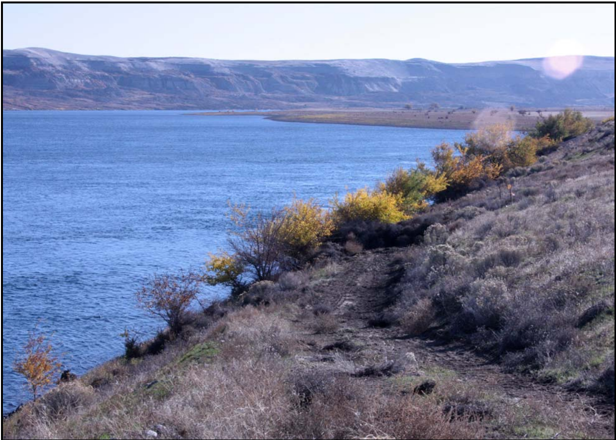
The project team removed brush from the road to 100-F-45, which contains buried riverbank effluent pipeline. (Photo 6)
