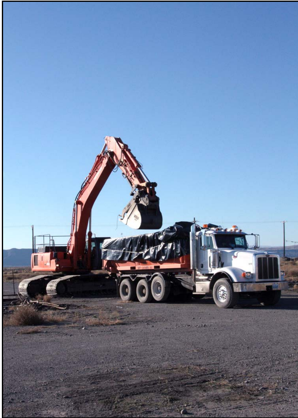
Washington Closure Hanford subcontractor Ojeda Business Ventures continues excavation and loadout at 100-F-44:8, a site that contains old fuel pipelines. (Photo 7)
