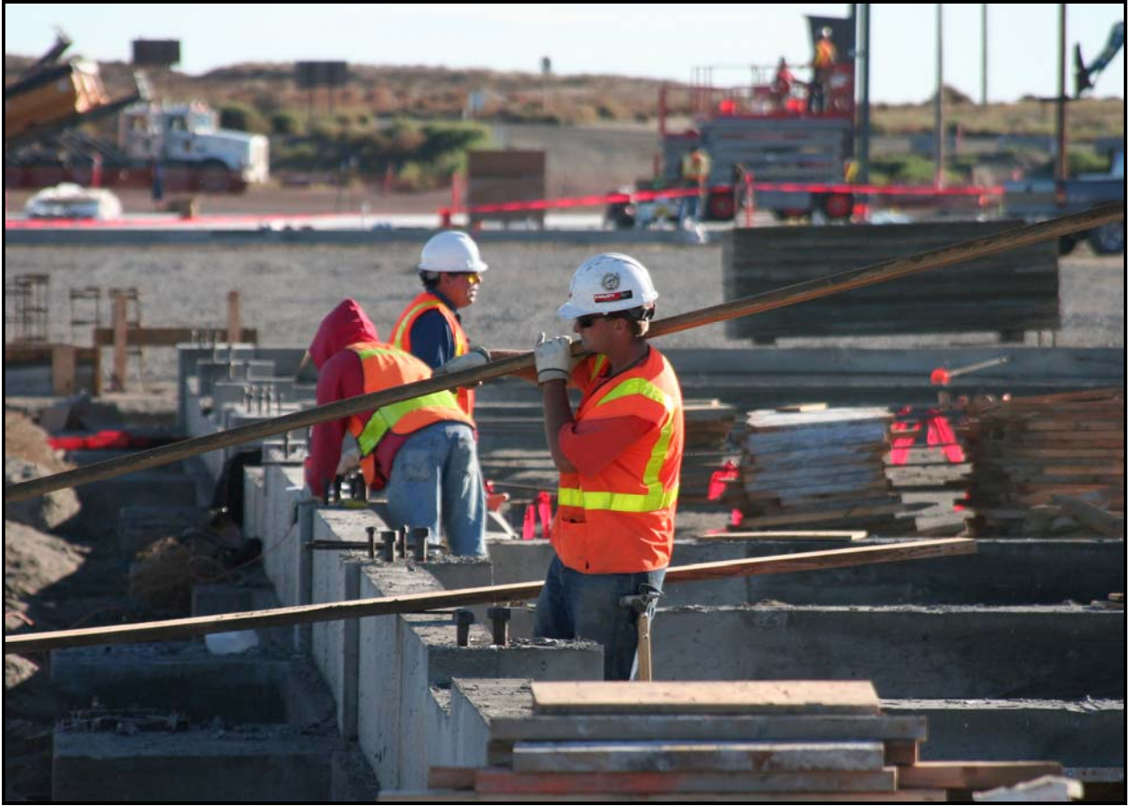
Workers from Fowler General Construction begin work on the underground utilities for the equipment maintenance facility/operations center at the Environmental Restoration Disposal Facility. (Photo 5)
