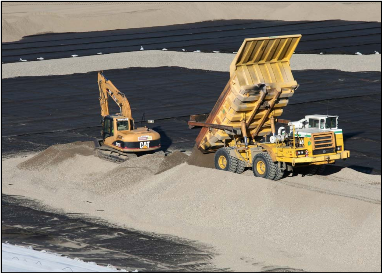
Washington Closure subcontractor TradeWind Services places the gravel drainage layer in super cell 10 at the Environmental Restoration Disposal Facility. (Photo 2)
