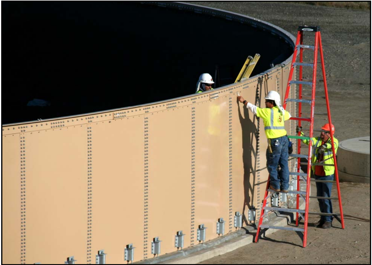
Workers continue to install the liner for leachate storage tank No. 3 at the Environmental Restoration Disposal Facility. (Photo 3)
