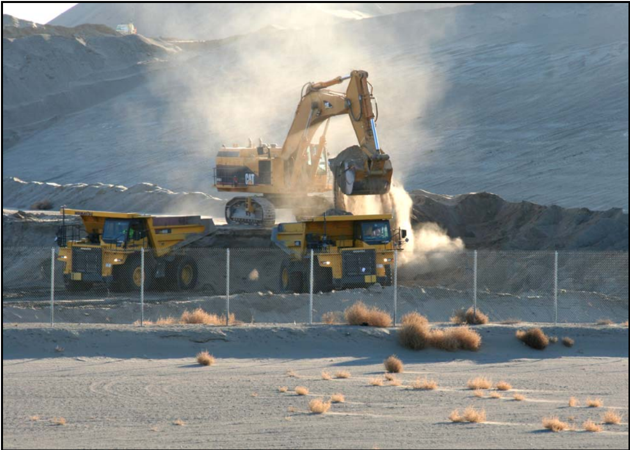
Excavation of super cell 9 continues at the Environmental Restoration Disposal Facility. More than 1.49 million cubic yards of dirt has been removed.
