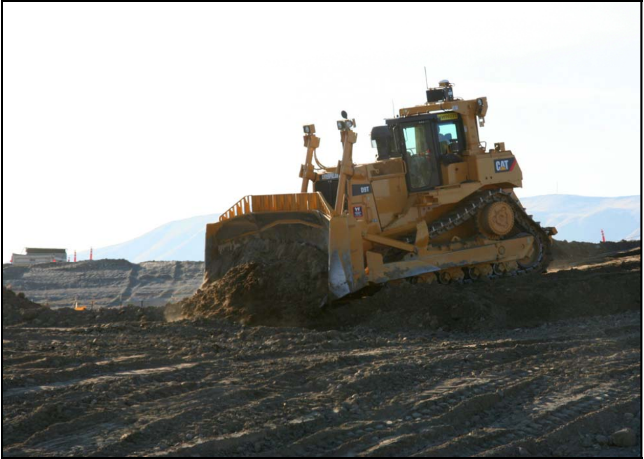
One of two D9 bulldozers recently delivered to the Environmental Restoration Disposal Facility clears dirt at the disposal site.
