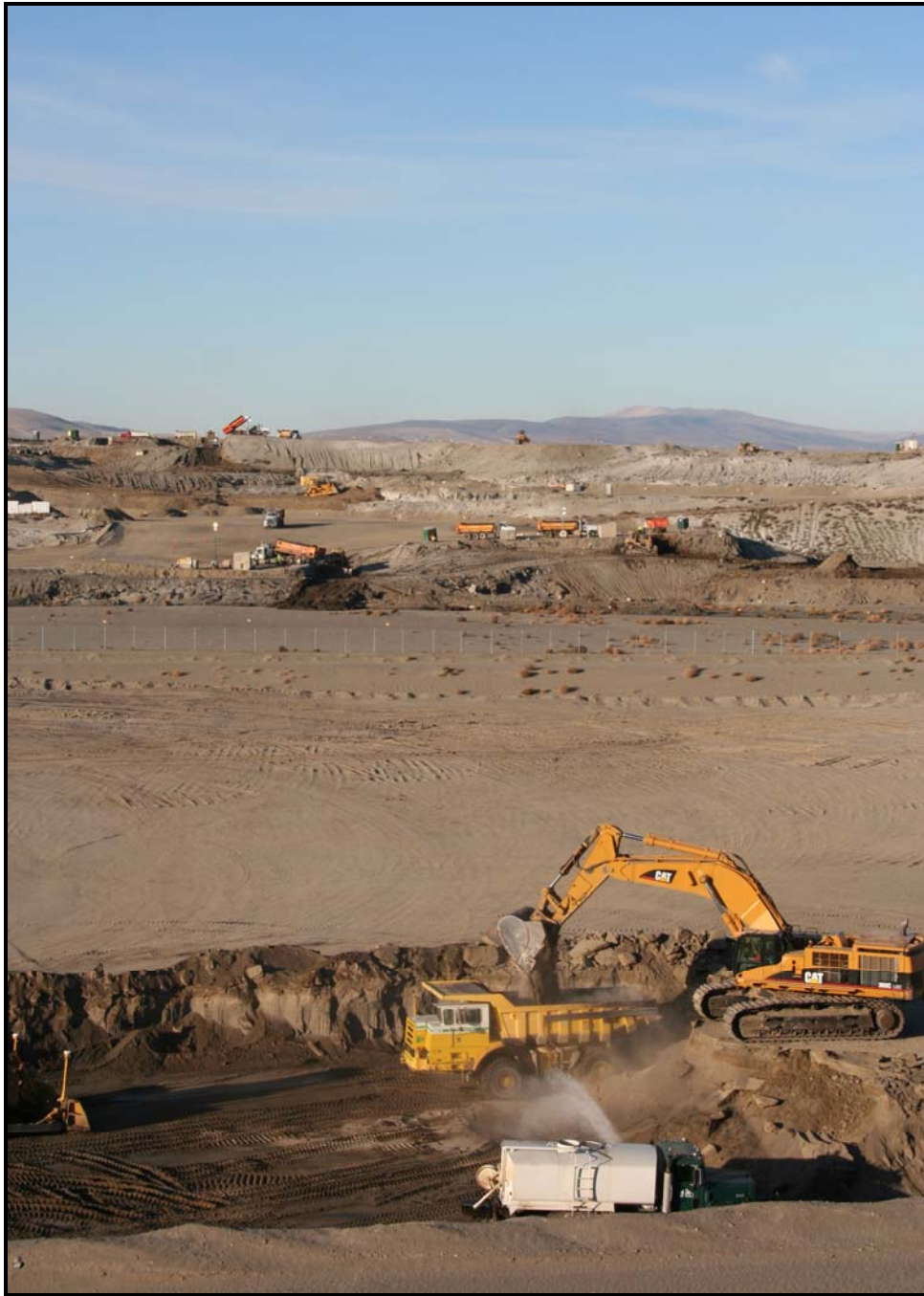
Excavation of super cell 9 at the Environmental Restoration Disposal Facility is expected to be completed in early February.
