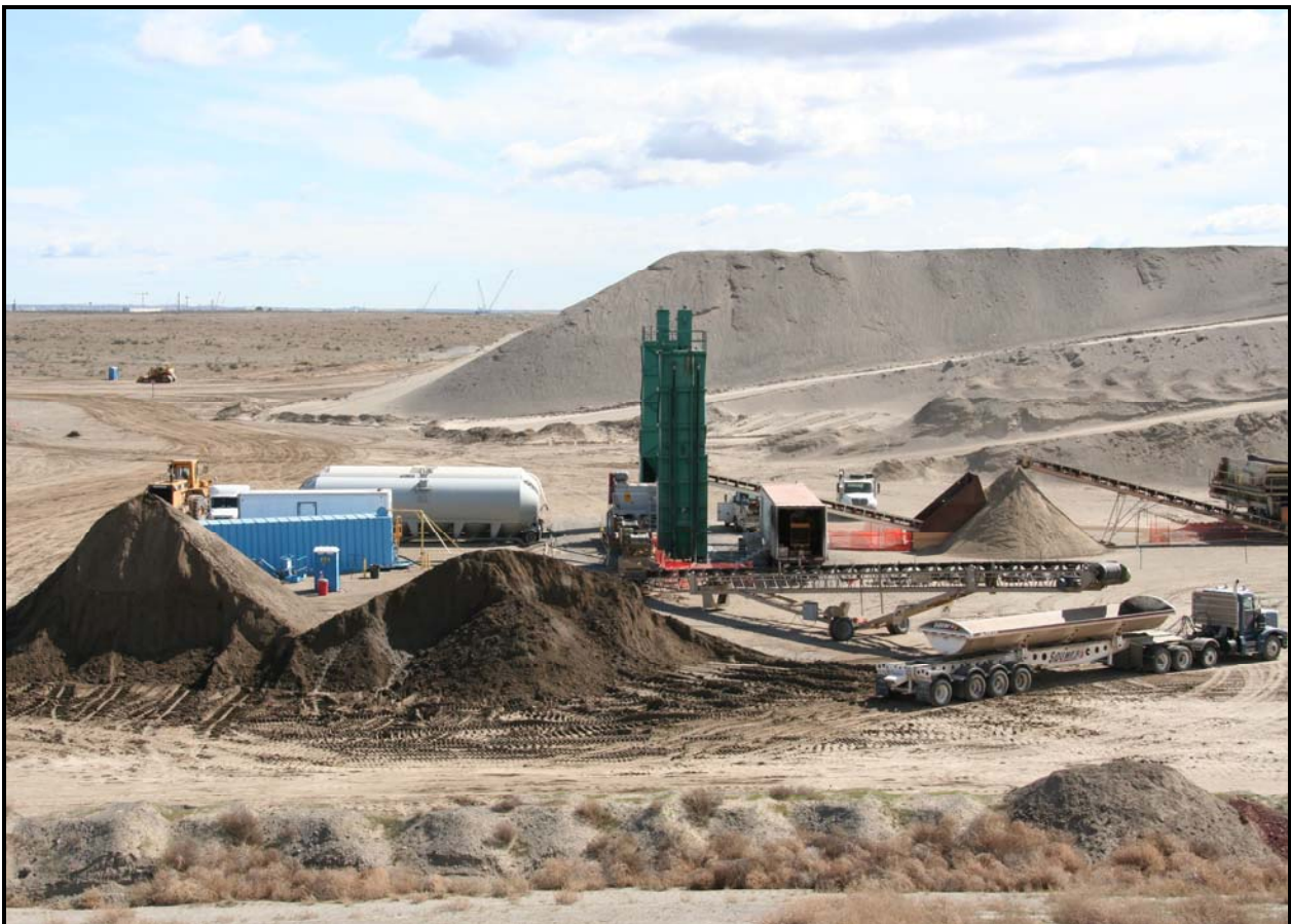
A pug mill is used to manufacture the soil/bentonite (admix) for the compacted soil liner to be used in super cells 9 and 10 at the Environmental Restoration Disposal Facility.
