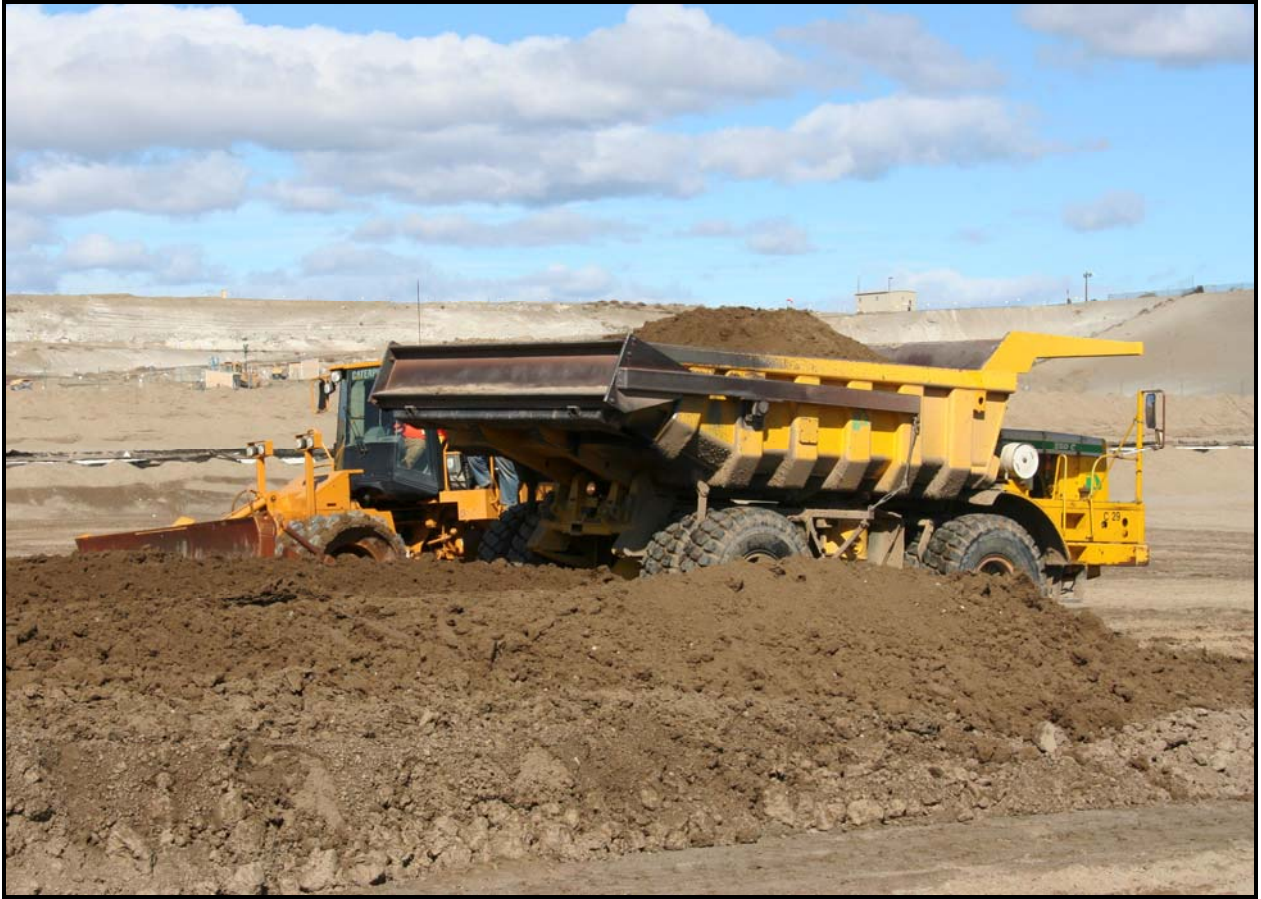
TradeWind Services personnel construct a test pad with the materials, equipment, and procedures that will be used to create the admix layer of the actual liner system.
