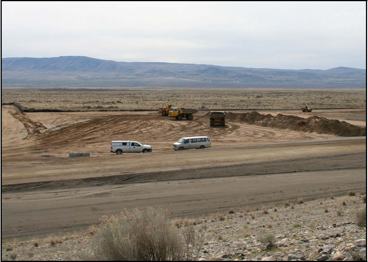
DelHur Industries grades the site for the expanded transportation yard at the Environmental Restoration Disposal Facility.
