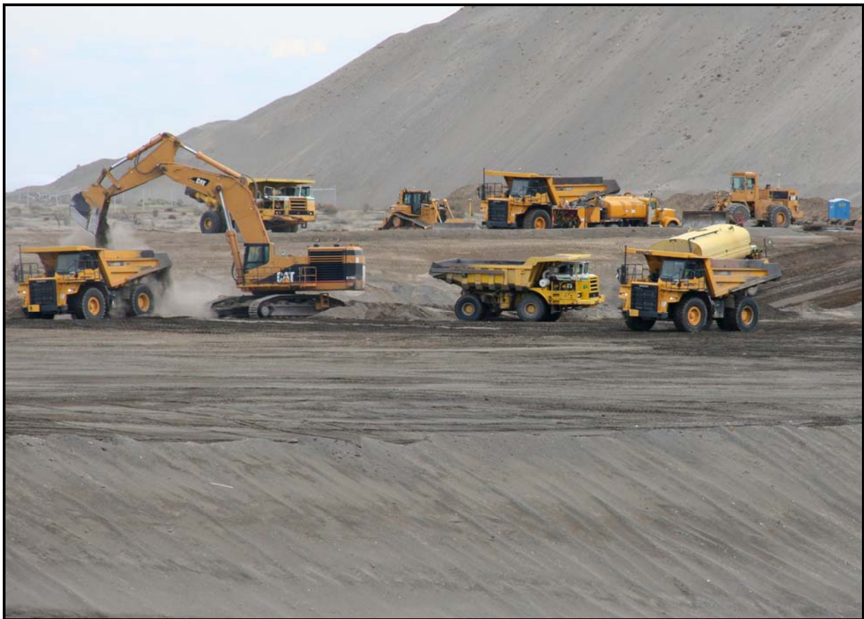
DelHur Industries has removed 405,115 cubic yards of soil from super cell 10 at the Environmental Restoration Disposal Facility.
