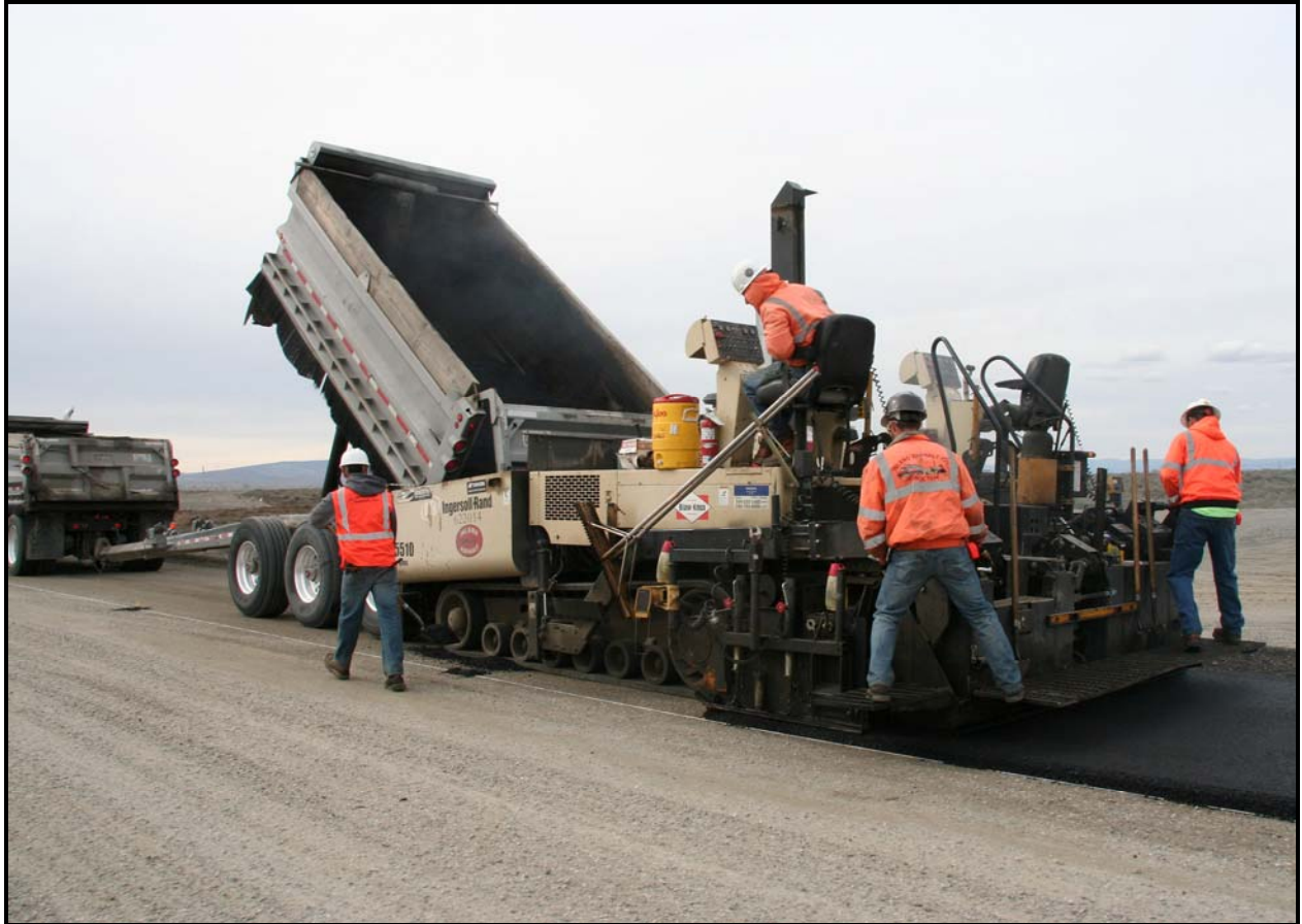
Inland Asphalt Co. lays asphalt on the back road to the Environmental Restoration Disposal Facility.
