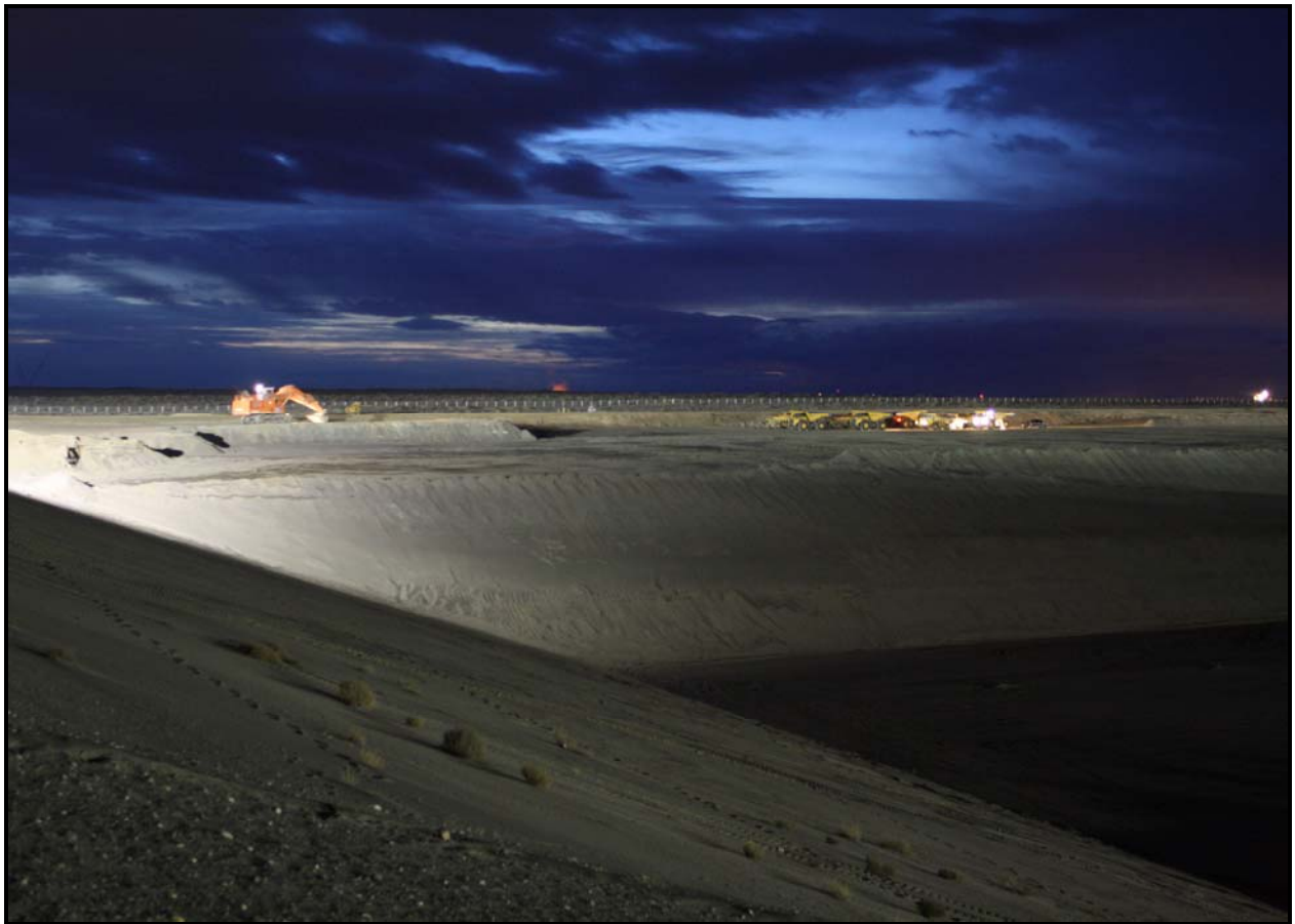
DelHur Industries gets an early start during excavation of super cell 10 at the Environmental Restoration Disposal Facility. This view is from the north end of super cell 9.
