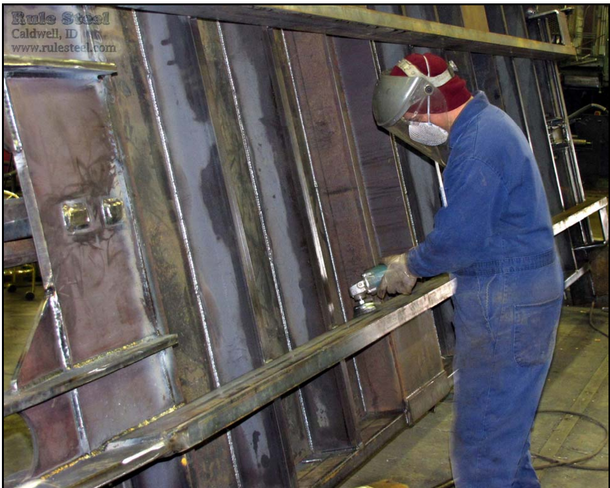
Rule Steel workers construct one of the 150 waste containers delivered to the Environmental Restoration Disposal Facility. Rule Steel is based in Caldwell, Idaho.
