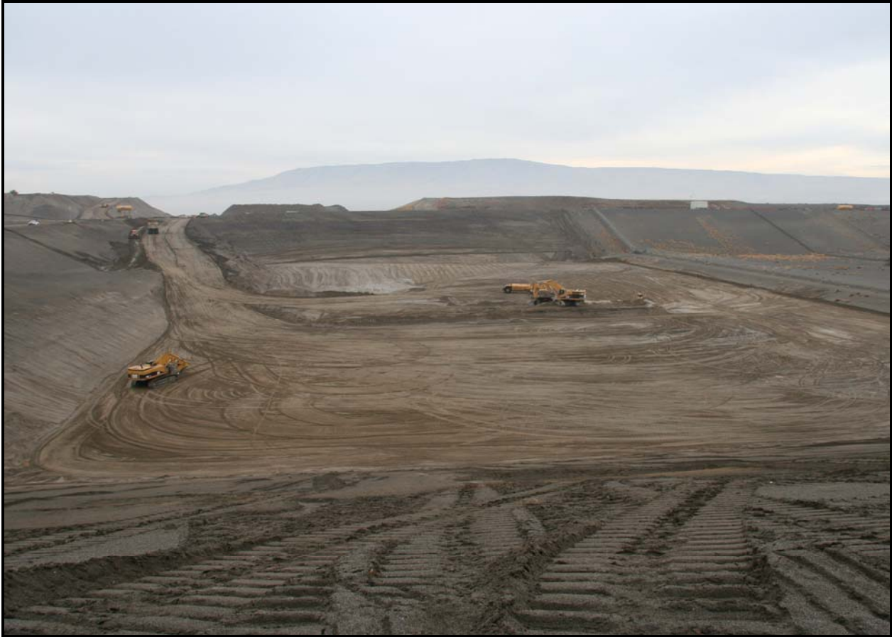
DelHur Industries personnel began excavating the south ramp, upper left, at the Environmental Restoration Disposal Facility.
