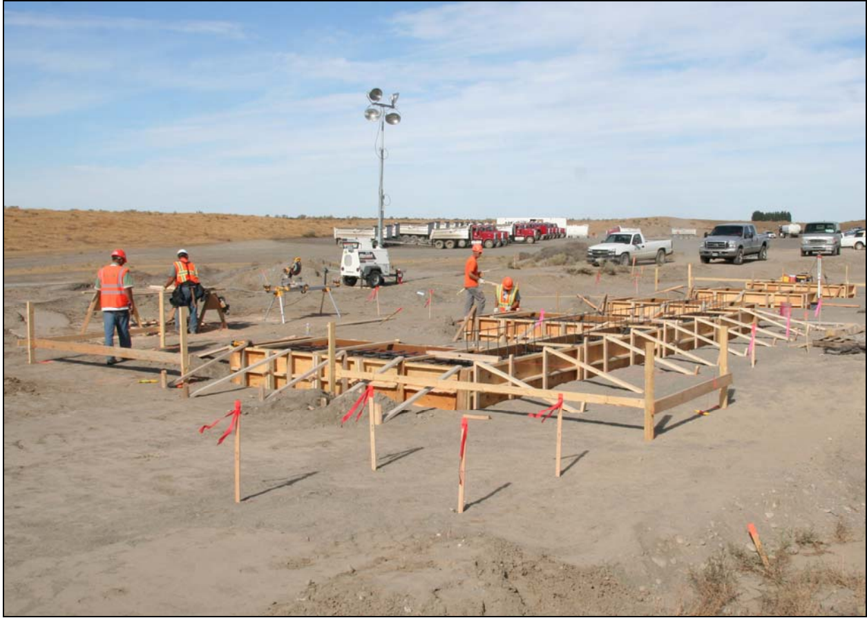
Workers prepare concrete forms for a new scale to support waste shipments into ERDF.
