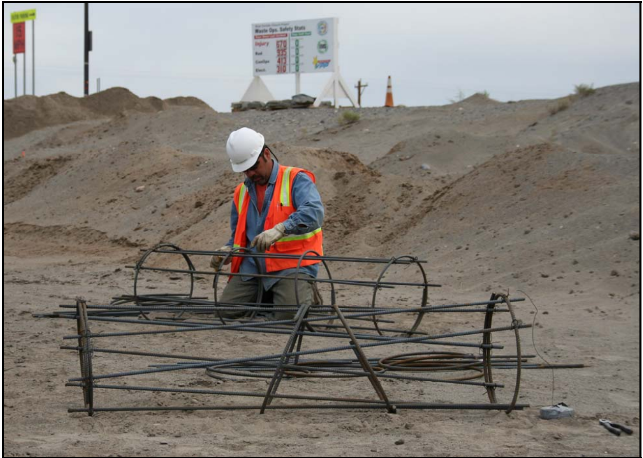
A worker prepares rebar cages for light pole installations near a new access road and container transfer area at ERDF.
