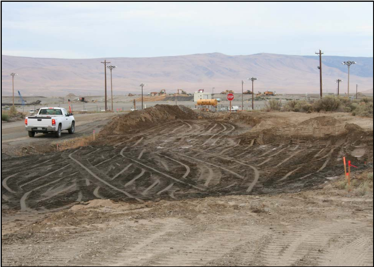
Site preparation is underway for a new scale that will accommodate the increasing volume of containers from other Hanford contractors and WCH.
