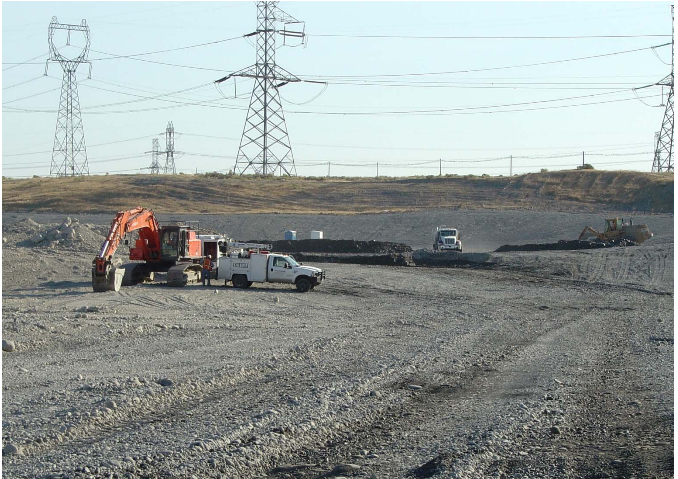
Workers performed site preparations for the temporary Container Transfer Area at the 100K Area. The area will support the waste site remediation that will be performed with the support of Recovery Act funds.
