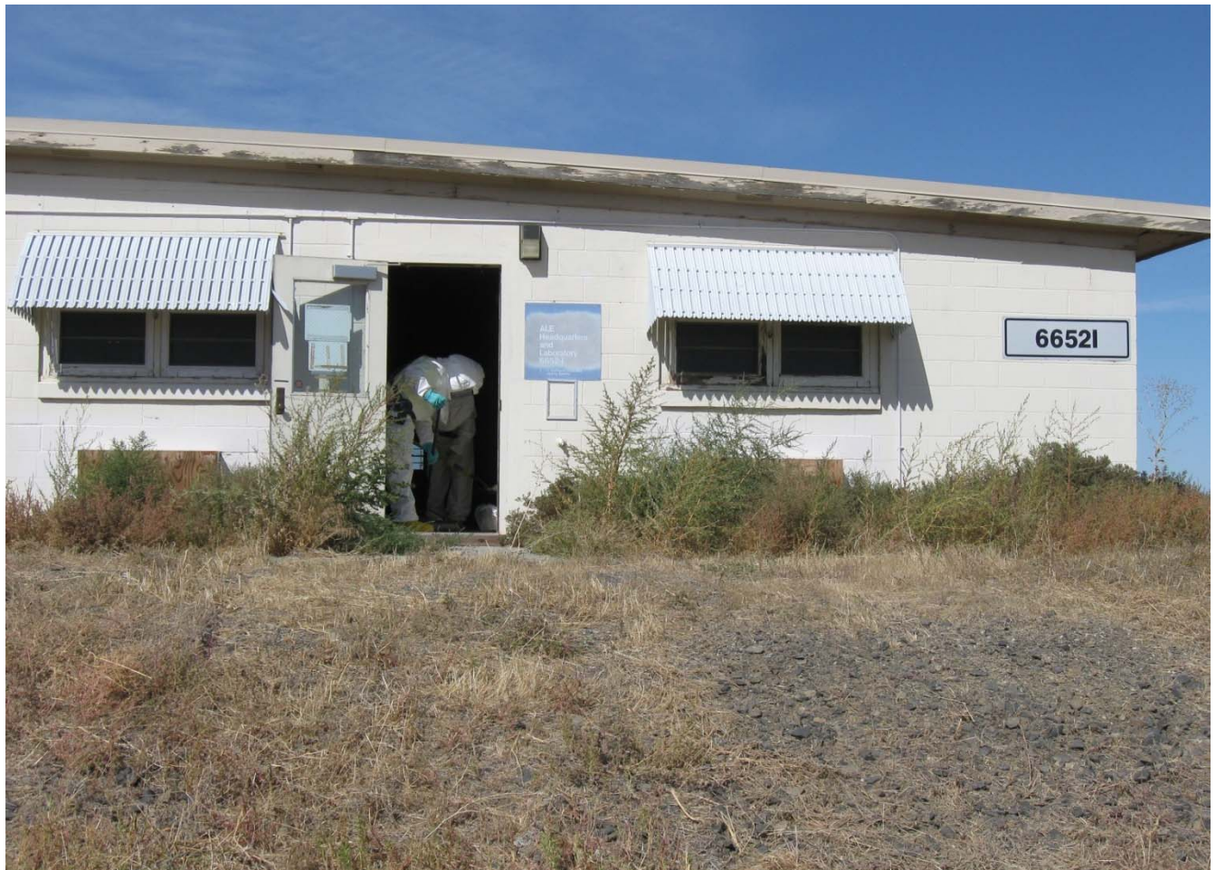
After confirmatory radiological surveys and biological cleanup were finished, buildings 6652-M, -H and -J were down-posted.
