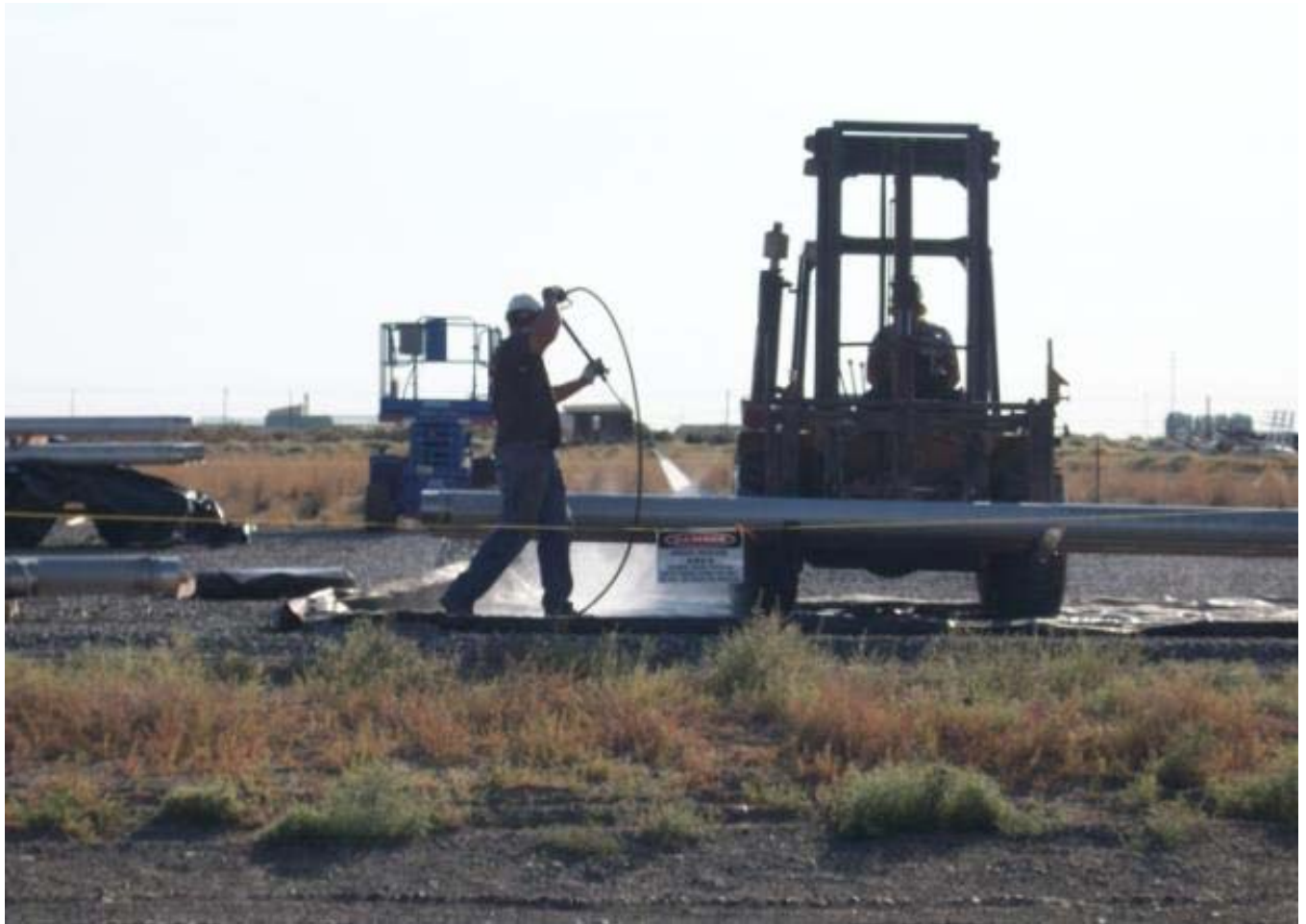
At the 200-ZP-1 site, workers from the subcontractor Blue Star clean a well casing prior to installation.
