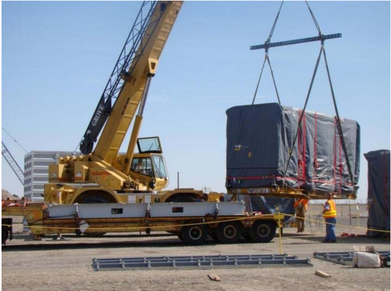
On Sept. 16, Box 29 was loaded out of 3A Trench 17. The box contains suspect TRU waste. Once removed from the trench, the box was placed upon a platform and covered with another shipping container for shipment to the CWC.
