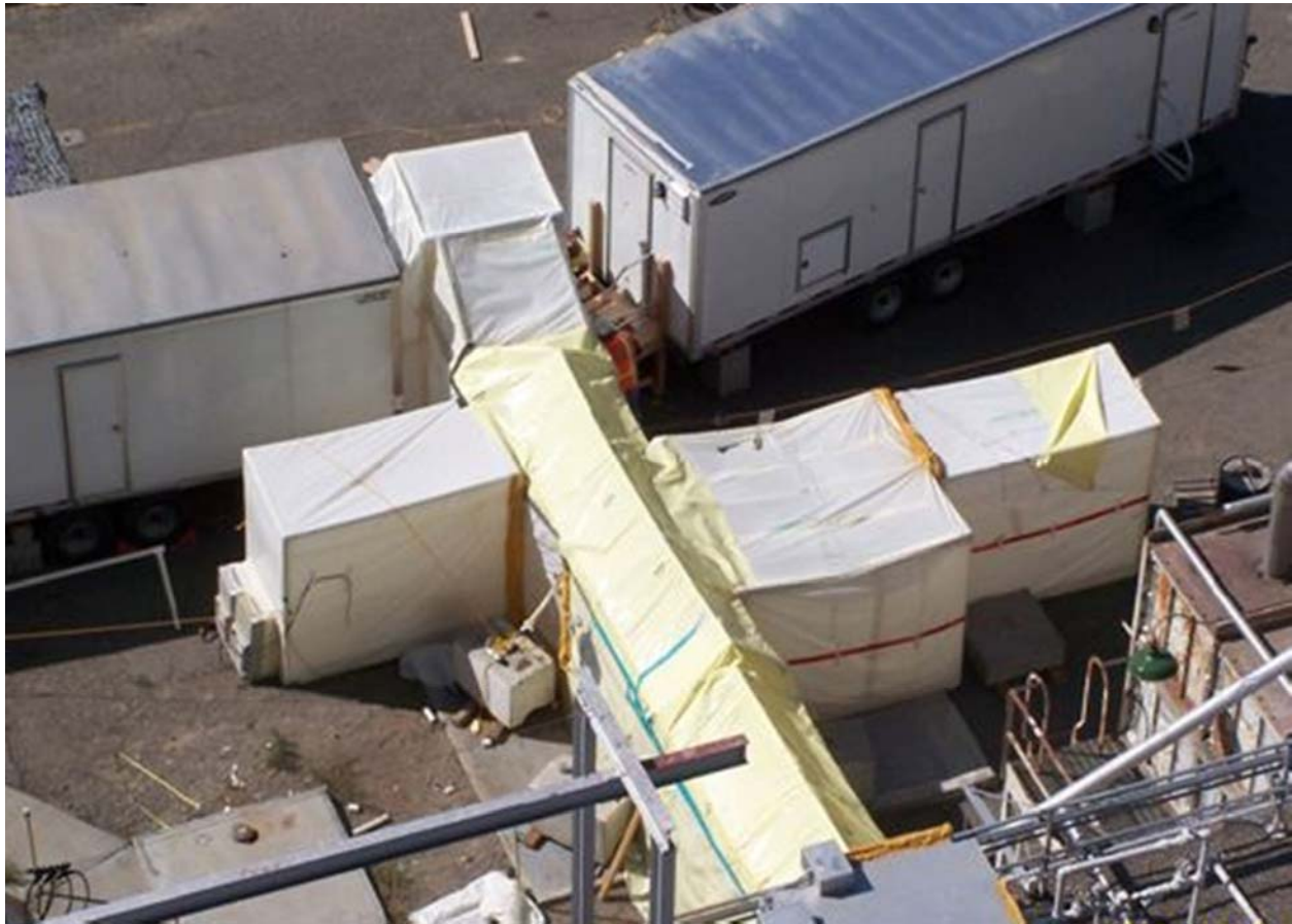
Construction of tunnels to the shower trailers for the asbestos abatement was completed at the 224-UA building.
