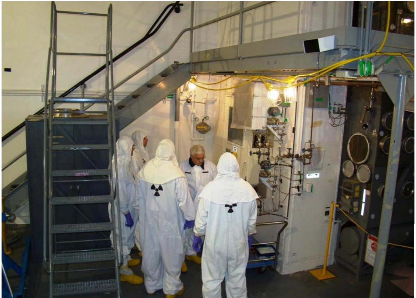
Workers conduct a walk-down for future removal of a glove box from room 232 in the 234-5Z building.
