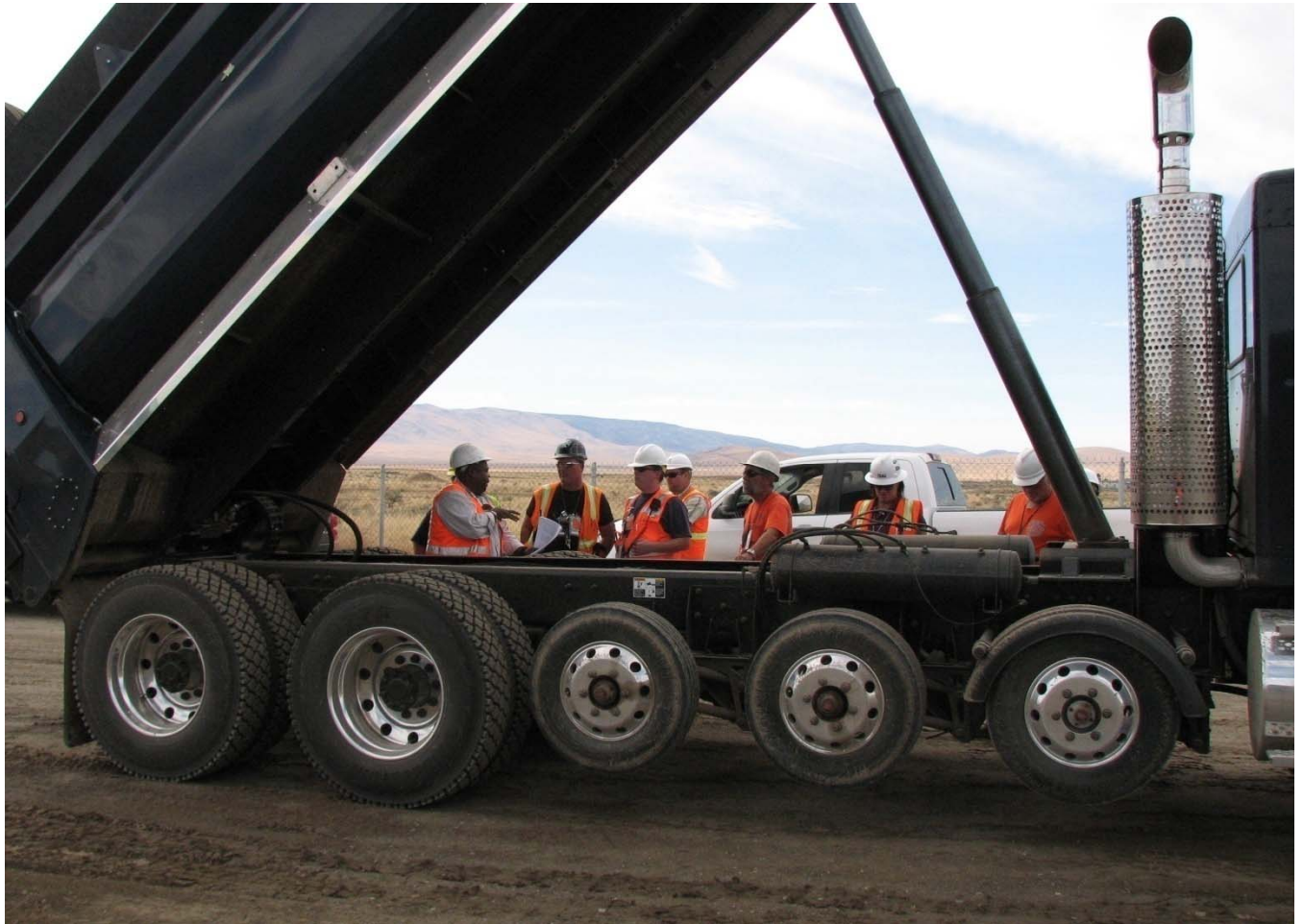
Workers were instructed in how to operate the recently procured dump trucks that will be used to facilitate remediation in the BC Control Area.
