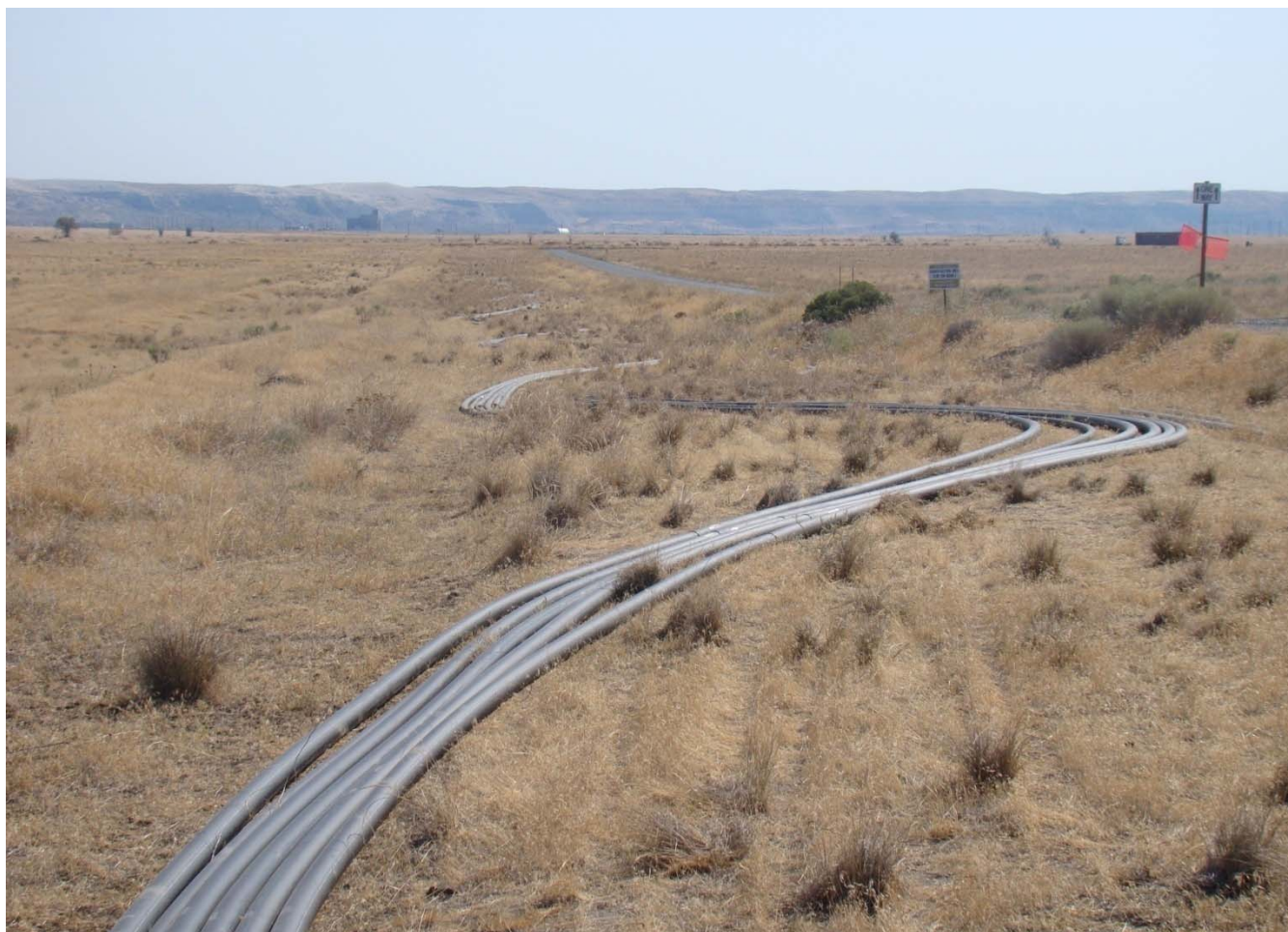
Out at the 100-HR-3 site, workers are laying several miles of HDPE pipe that will expand the 100-HR-3 area groundwater treatment system. Laying the pipe includes heat bonding sections of the pipe together, which workers have done without incident.
