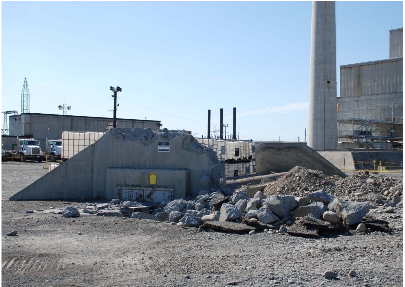
Shielding was removed and demolition continued on the 118KE Horizontal Control Rod Storage Cave, shown here with additional materials awaiting disposal. Removing the shielding will allow for removal of the cave mouth and tubes.
