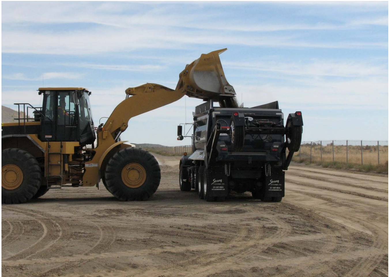
After observing demonstrations from trained personnel on how to operate the equipment, workers practiced operating the machinery.
