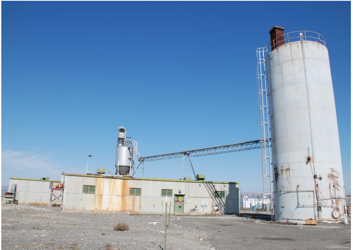
A walk down was performed on the 183KW Water Treatment Head House to identify asbestos for removal. After the asbestos is removed the facility will be available for demolition as part of the sedimentation basin removal project.
