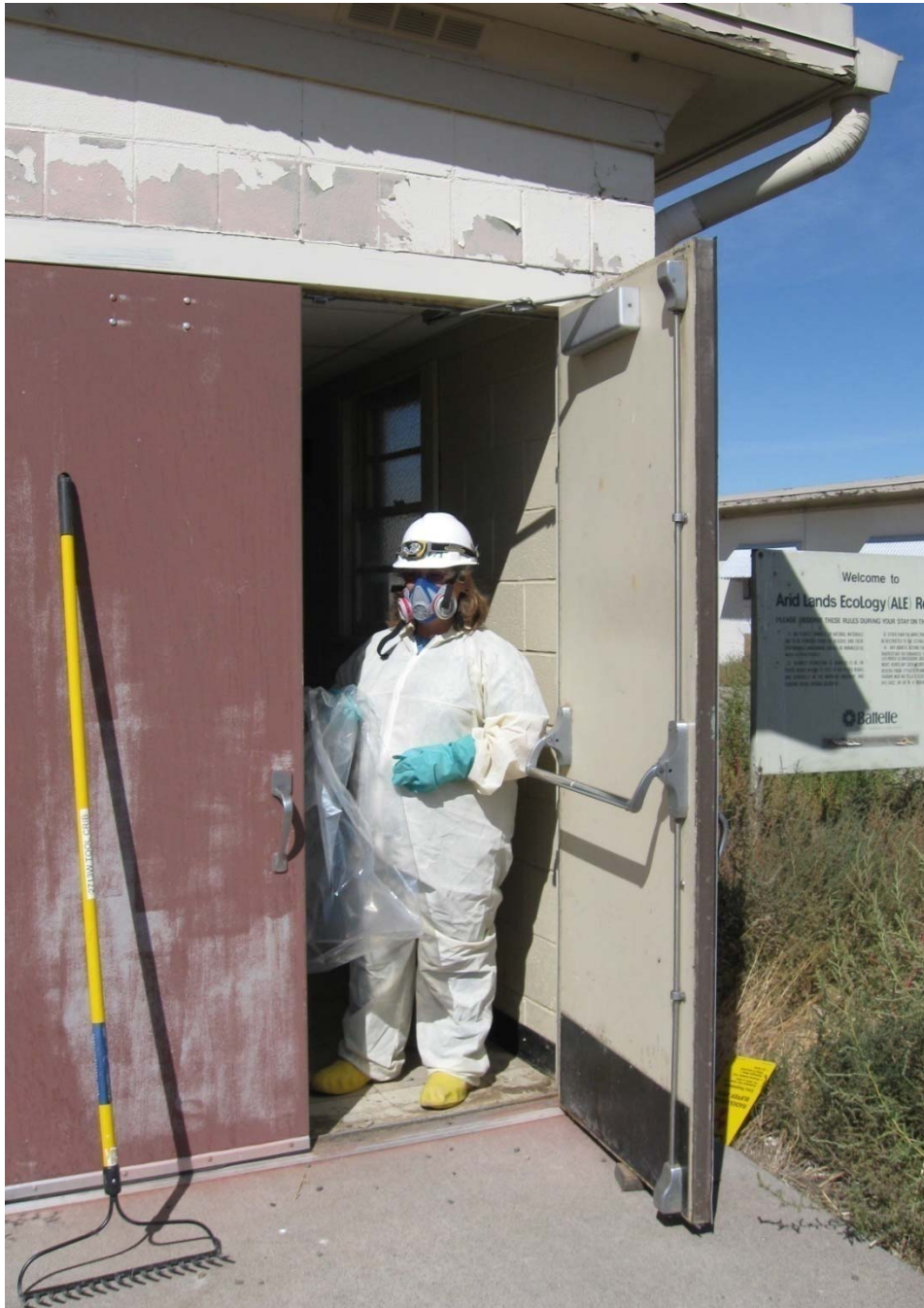
A worker performs biological cleanup at the Lower ALE facilities, where work is beginning to prepare the facilities for demolition.
