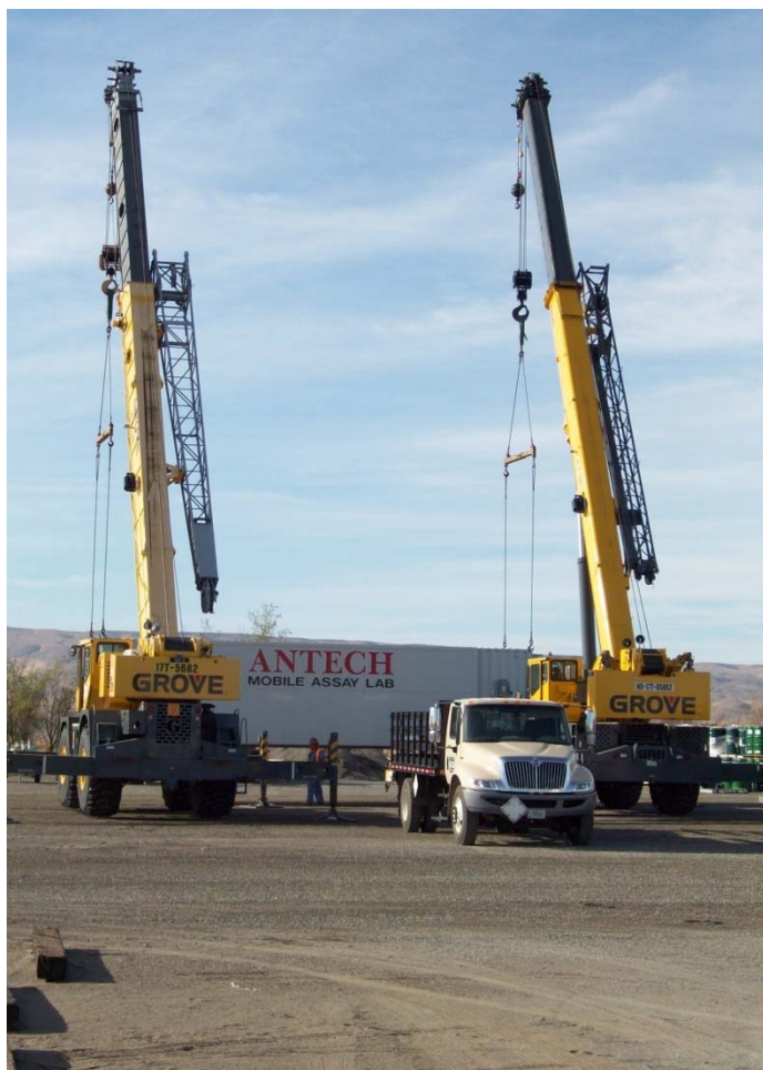
During the week ending Sept. 18, demobilization on the ANTECH Mobile Assay Lab was completed and the lab was crane-lifted onto a Hanford tilt trailer and transferred to a commercial vehicle.
