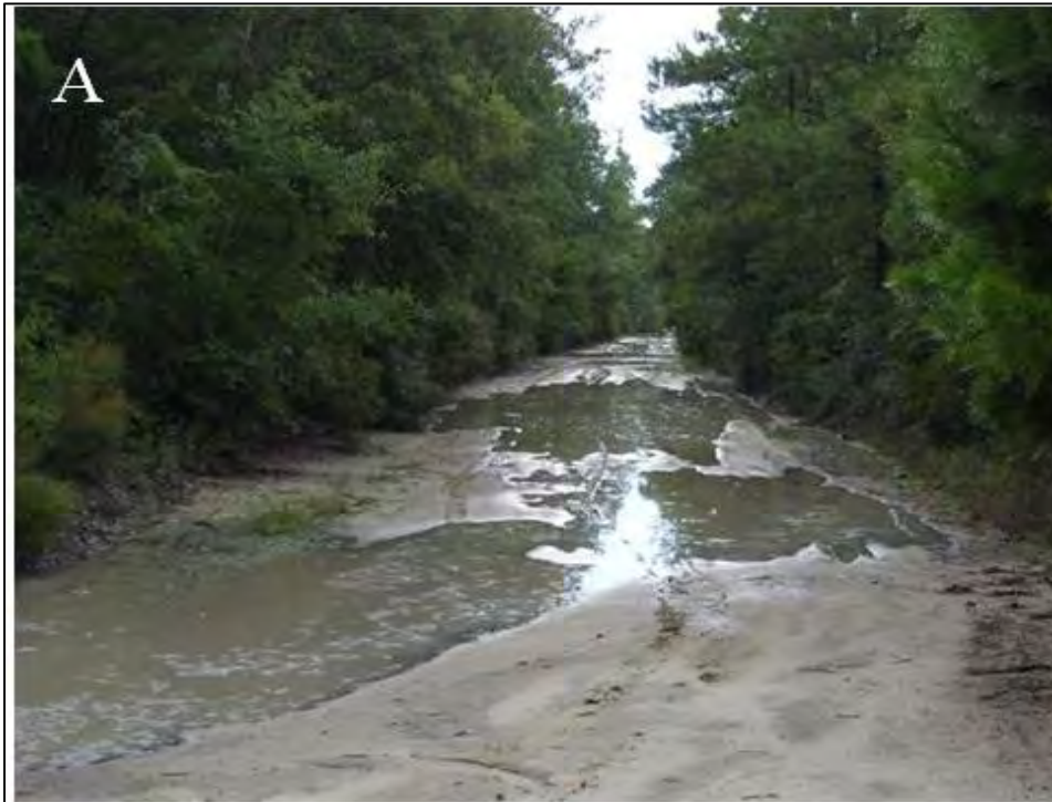
Figure 31. Comparison of unpaved road condition before (A) and after (B) restoration at Dripping Rock. Photo credit: The Nature Conservancy.
