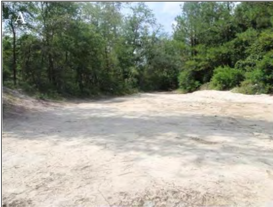
Figure 33. Comparison of condition of the unpaved road terminus at the breached riverbank, facing west along the riverbank, before (A) and after (B) restoration at Dripping Rock. Photo credit: The Nature Conservancy.
