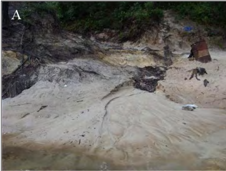
Figure 36. Comparison of condition of the breached riverbank, looking up-slope from the Yellow River, before (A) and after (B) restoration at Dripping Rock. Phot credit: The Nature Conservancy.
