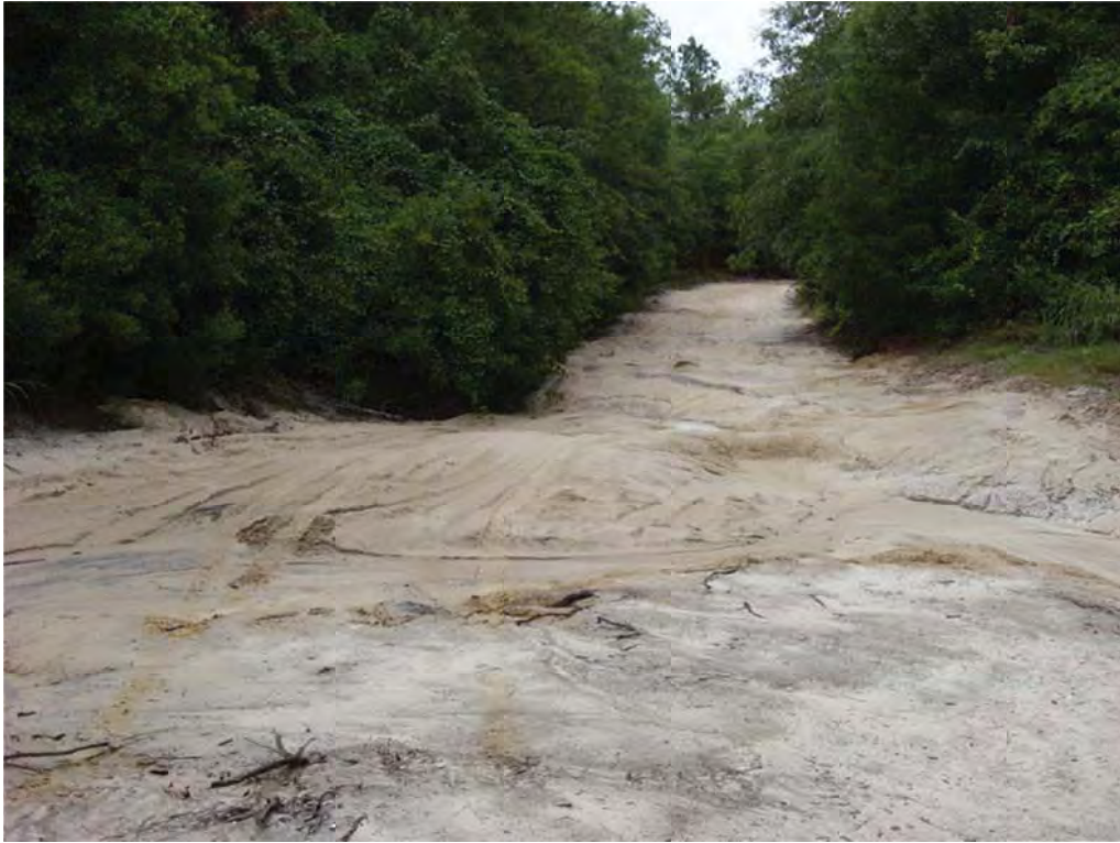
Figure 5. Eroding unpaved road discharging into the Dripping Rock site, Yellow River.
