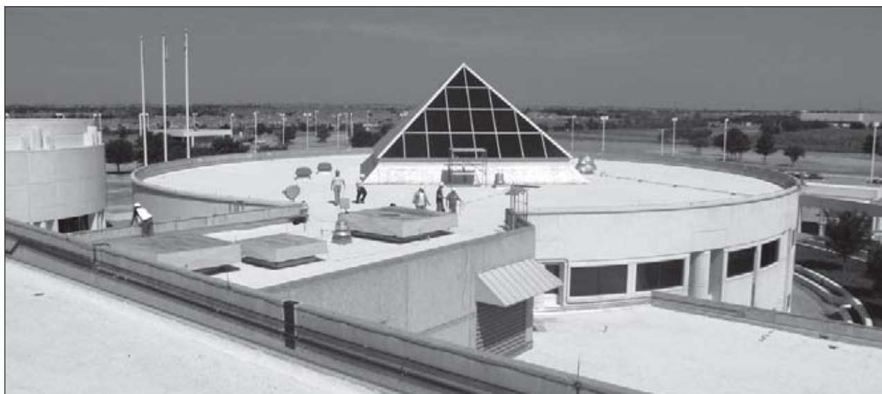
Workers put finishing touches on a cool roof area around the WCF pyramid.
