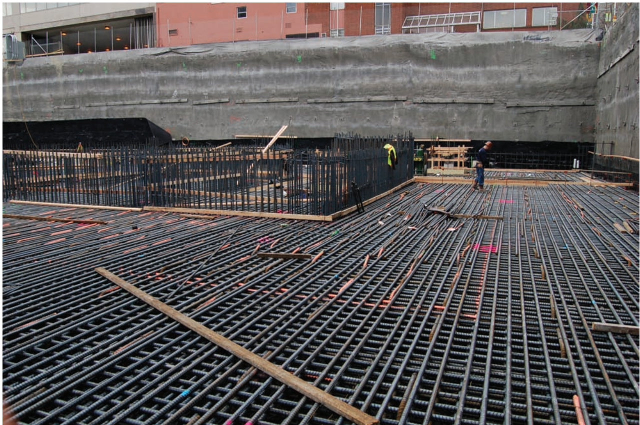
Figure 10-2 – Mat foundation under construction, 90° hook shear reinforcement (painted orange) being placed from above.
