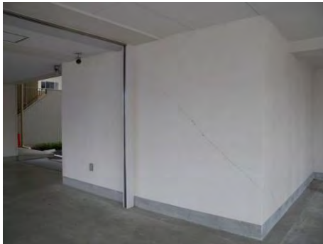
Photo 3.74 Shear Crack on the Wall
