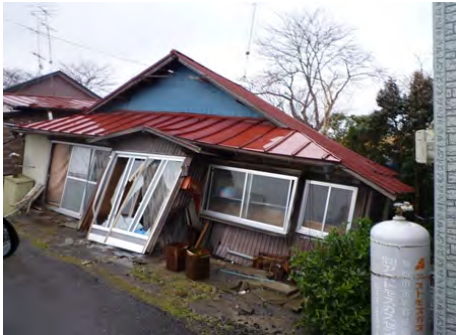
Photo 3.1 Damage of Houses caused by Ground Transformation
