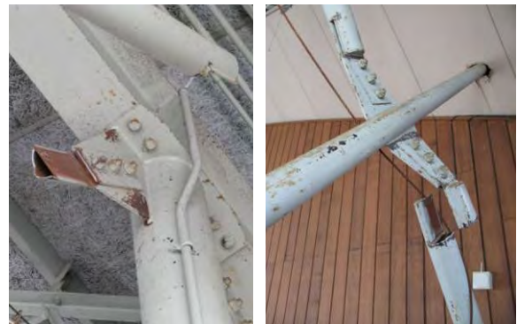
a) Fracture at column top b) Fracture at brace crossing Photo 3.49 Fracture of Brace Welded Connection
