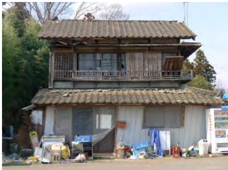
Photo 3.19 Damaged House with Shop
