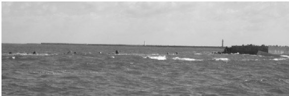
Fig. 5 Damaged north breakwater in Hachinohe Port
