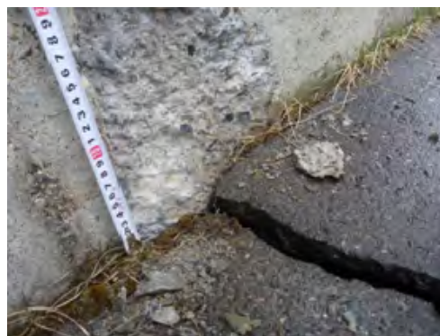
(b) Level difference at joint
