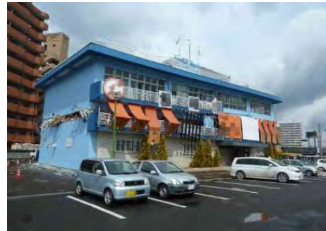
Photo 3.23 Mid-story Collapsed Building
