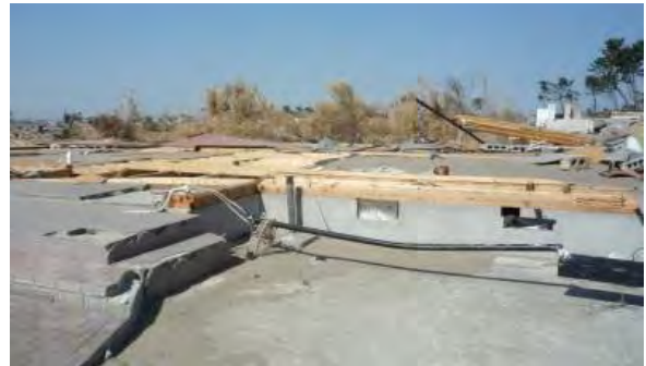
Photo 4.13 Remaining Ground Sill after Washout of Superstructure
