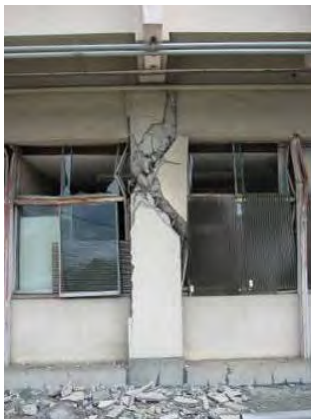
Photo 3.26 Shear Failure of Column
