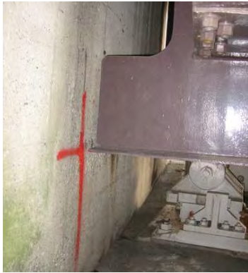
(a) Shortened Deck-end Gap Resulting from Movement of Abutment
