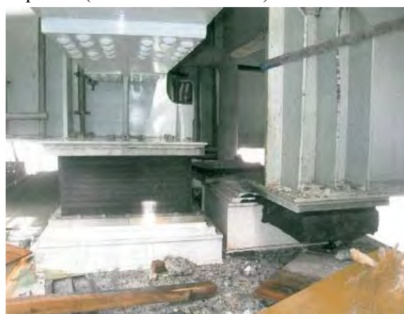
Photo 11 Transverse offset of a girder due to rupture of elastomeric bearings
