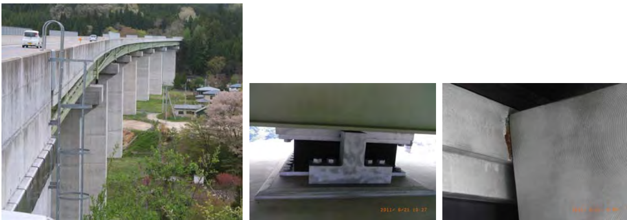
Photo 3 Yamada viaduct and its bearing. The top plates of bearings were scraped by the side blocks.
