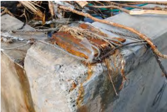
Photo 22 Failure of a RC side stopper, and four steel stoppers for preventing excessive longitudinal deck response which were not damaged
