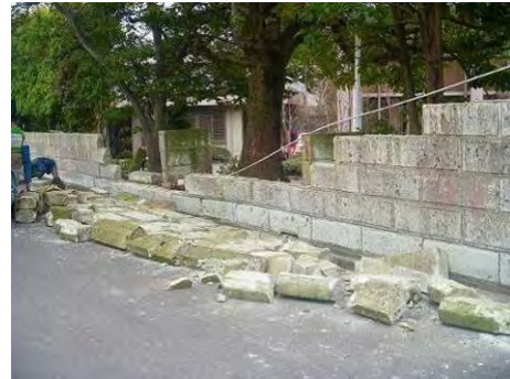
Photo 3.46 Collapse of Stone Masonry Wall
