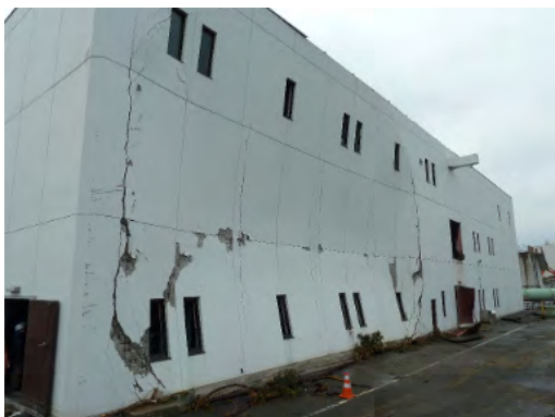
Photo 4.5 Out-of-plane Fracture of Reinforced Concrete Shear Wall without Floor
