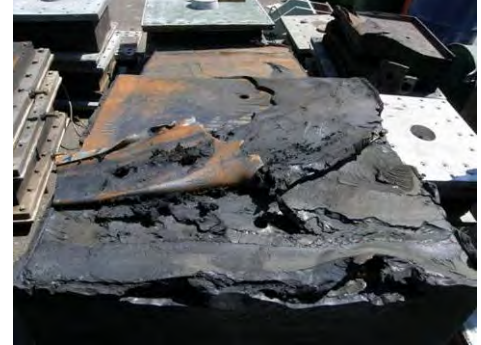
Fig.8(4) Rupture of Rubber Bearing (April 6)
