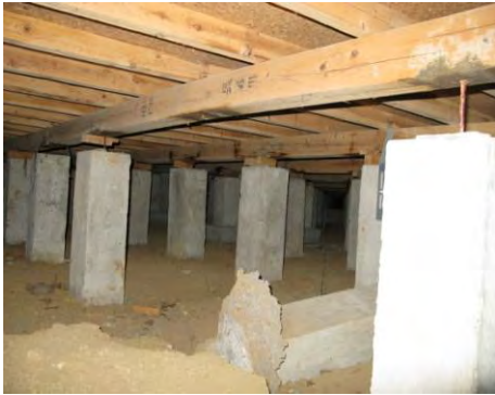
Photo 3.55 Overturning of Floor Strut
