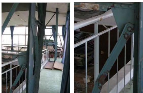
a) Latted column b) Buckling of diagonal member Photo 3.51 Buckling of Diagonal Member of Latted Column
