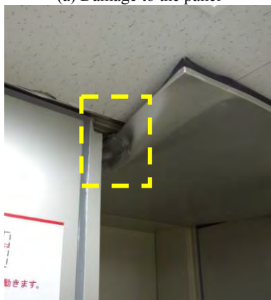
(b) Damage to the expansion joint
