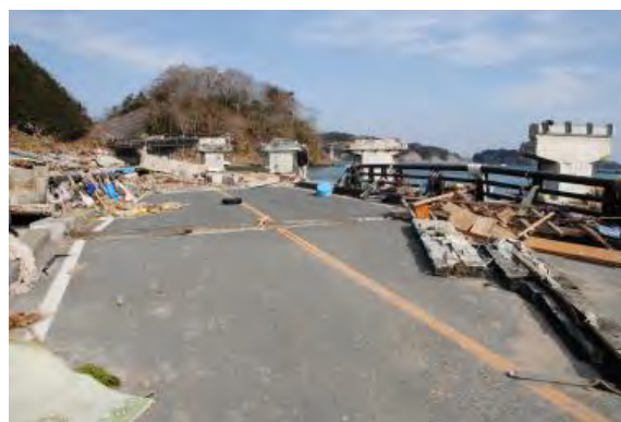
Photo 18 Damage of Utatsu Bridge
