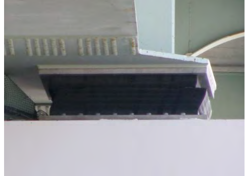
Fig.8(3) Rupture of Rubber Bearing on Pier No.54 (April 6)
