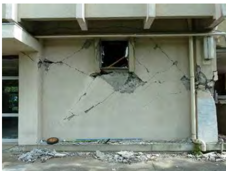
Photo 3.27 Shear Failure of Wall with Opening
