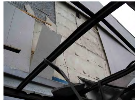
Photo 3.60 Falling of Exterior Finish Materials
