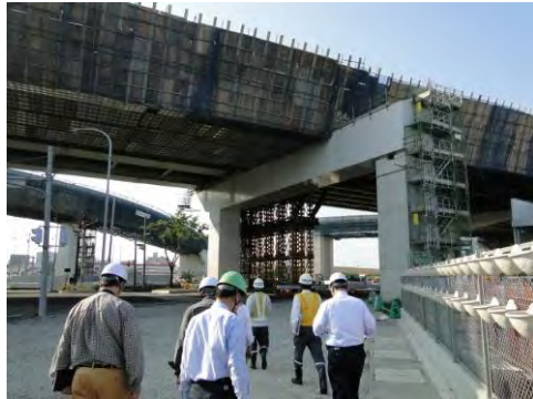
Fig.8(1) Sendai-Tohbu Viaduct (June 3)
