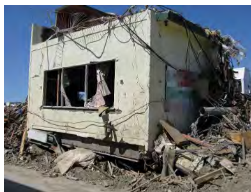
Photo 4.1 Story Collapse of 2-story Reinforced Concrete Building
