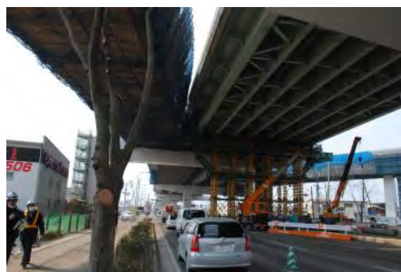
Photo 10 Piers where elastomeric bearings ruptured (Sendai-Tobu viaduct)
