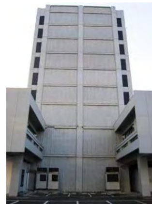
Photo 3.28 Appearance of Damaged Building
