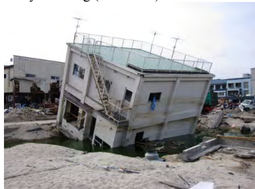
Photo 4.4 2-story Reinforced Concrete Building that was Tilted by Scouring
