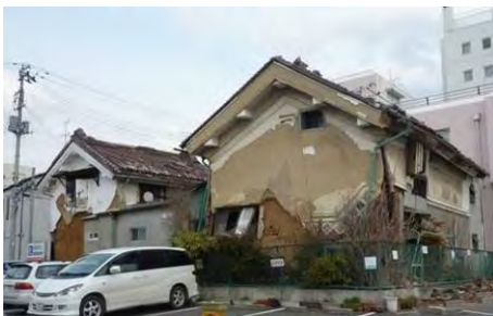
Photo 3.14 Dozo with Residual Deformation
