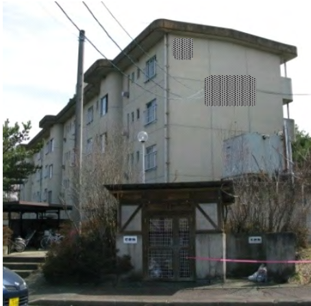
Photo 3.34 Appearance of Sank and Leaned Building
