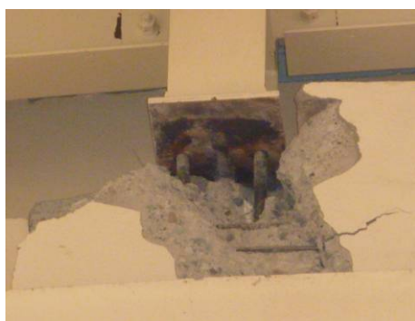
Photo 3.52 Spalling of Concrete
