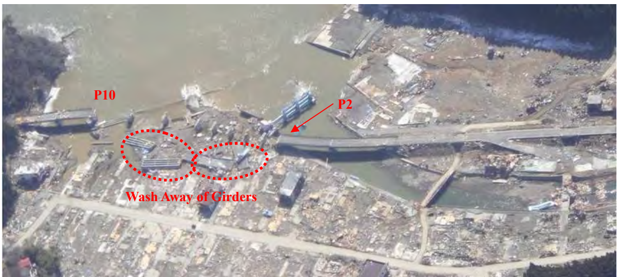
Fig.7(3) Utatsu Ohashi Br. (March 19, provided from Tohoku Regional Development Bureau, MLIT)
