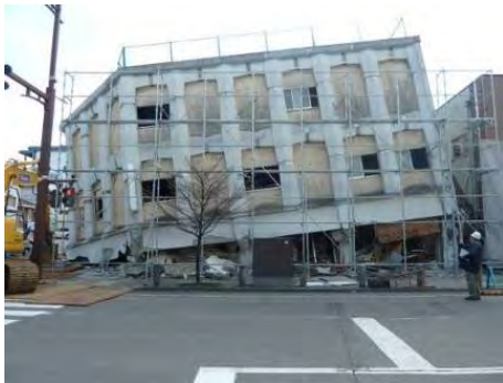
Photo 3.21 First-story Collapsed Building
