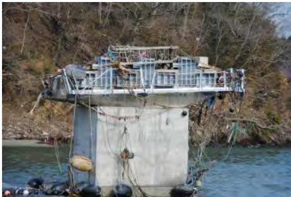
Photo 21 Steel devices for extending seat length (short device) and steel stoppers for preventing excessive longitudinal deck response due to ground motions (tall device)
