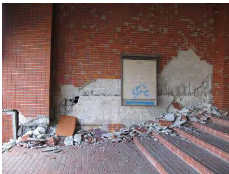
Photo 3.30 Damage on the Bottom of SRC Column and Shear Wall
