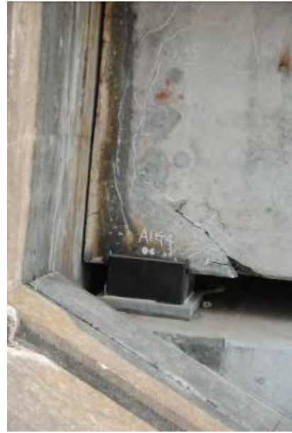
Photo 4 Damage of PC girders near the support
