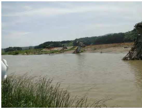
Fig.4(3) Collapsed Railway Bridge Columns near Koizumi Ohashi Br. (June 4)
