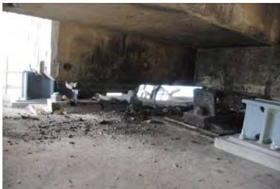
Photo 3 Damage of pin and roller bearings
