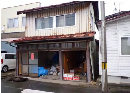
Photo 3.2 Damage of Houses with Store
