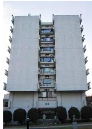
Photo 3.32 Appearance of Damaged Building
