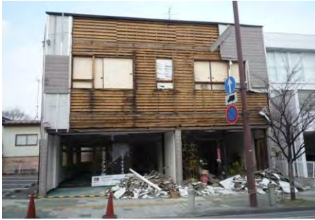
Photo 3.12 Fallen Mortar of Wall (Wood House with Shop)
