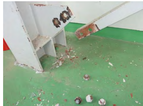
Photo 3.50 Fracture of Bolts
