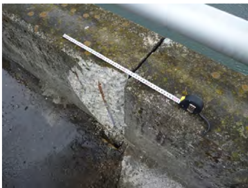
(a) Exfoliation of parapet concrete
