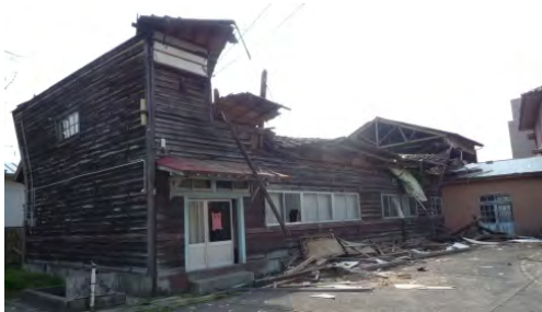
Photo 3.7 School Building whose 2 nd Story Collapsed
