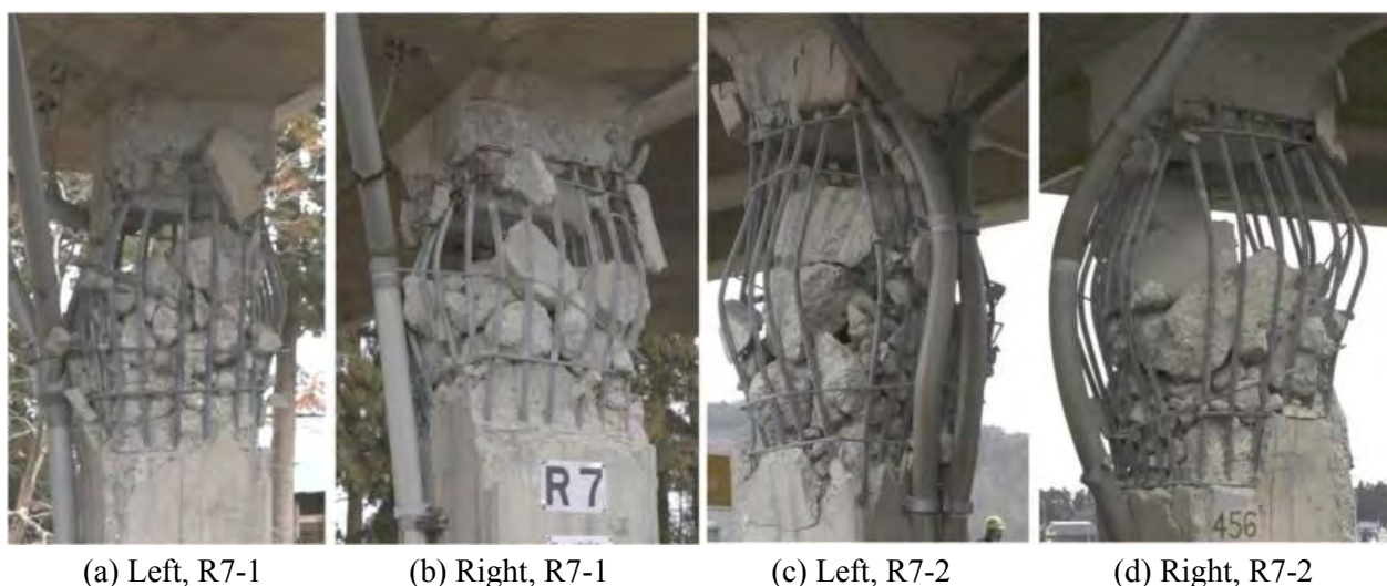
Photo 17 Close view of damage of R7-1 and R7-2 columns
