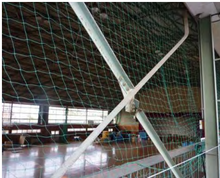
Photo 3.47 Buckling of Brace
