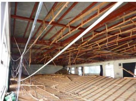
Photo 3.57 Dropping of Ceiling Materials
