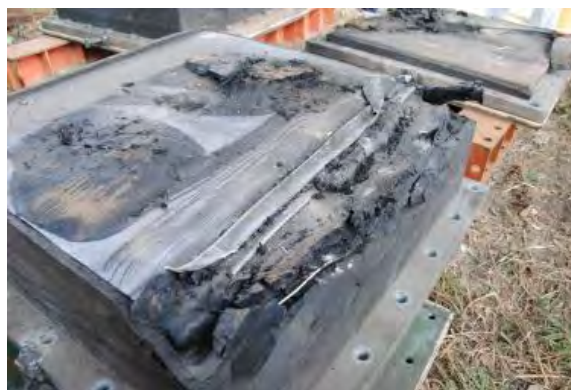
Photo 12 One of elastomeric bearings ruptured
