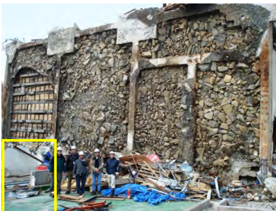
Figure 3 The ASCE Tohoku Tsunami Reconnaissance Team at the Onagawa uplifted and overturned 2-story reinforced concrete cold-storage building - Note low wall with top edge spalled (Hideyuki Kasano)
