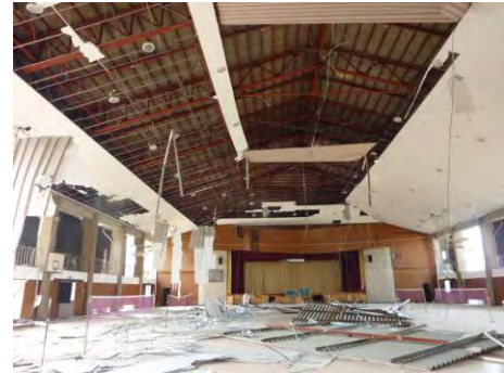
Photo 3.58 Dropping of Ceiling Materials
