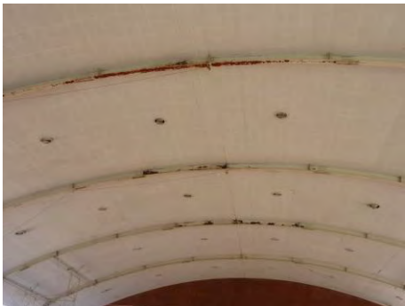
Photo 3.56 Peeling of Paints of Beam
