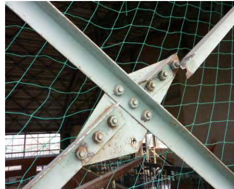
Photo 3.48 Net Section Fracture at Bolt Hole
