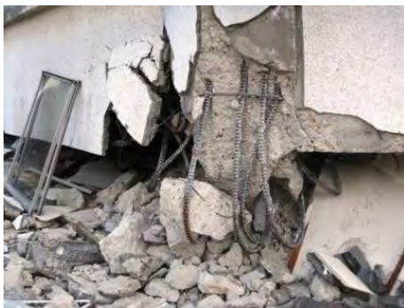
Photo 3.22 Close-up View of the Fallen Story
