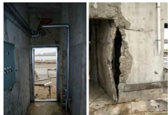
Figure 2: Wall corner joint and flexural failure by internal hydrodynamic pressurization
