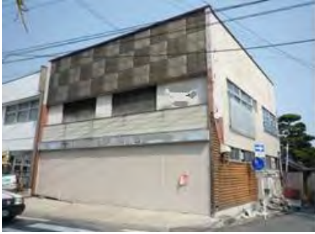
Photo 3.6 Store Combined House with Story Deformation
