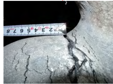
Photo 3.77 Lead Damper and Crack on the Surface
