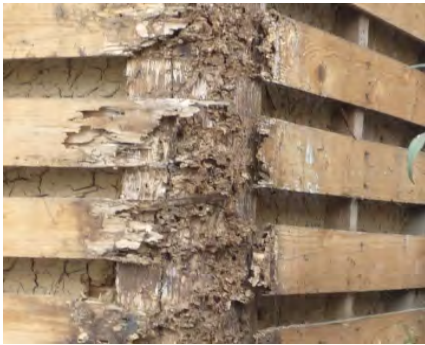
Photo 3.13 Bio-deterioration of Column and Based Mortar
