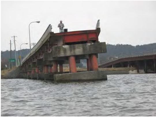
(a) Collapse of Bridge with Pile-bent Columns
