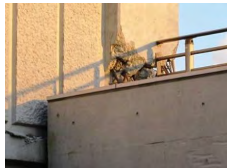
Photo 3.29 Crushing at the Bottom of Column on the Multi-story Shear Wall
