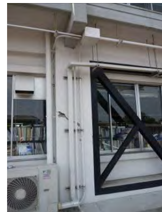
Photo 3.38 Shear Crack on Column with Framed Steel Braces
