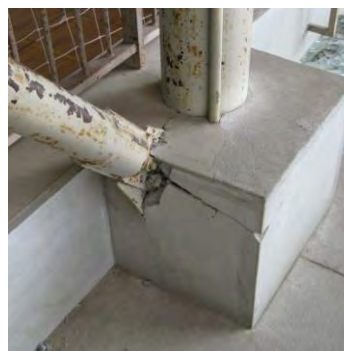
Photo 3.54 Cracking of Column Base Concrete
