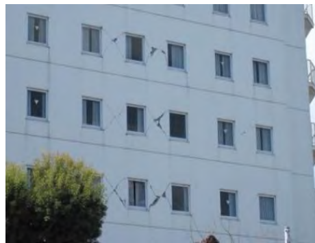
Photo 3.42 Shear Crack on Nonstructural Wall
