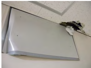
(a) Damage to the panel
