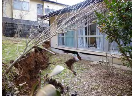
Photo 3.9 Damage of House
