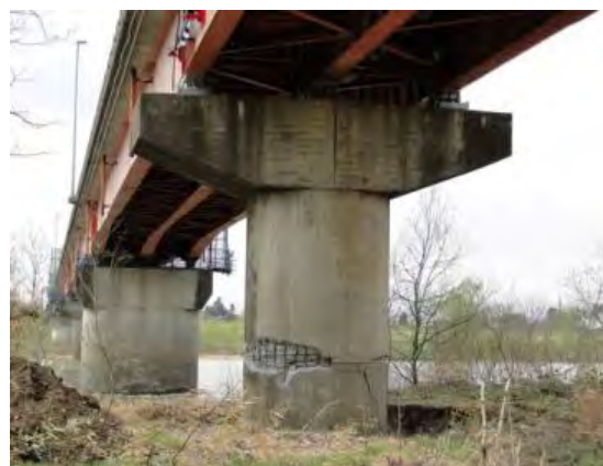
Photo 1 Shear failure of a column due to termination of longitudinal bars with insufficient development (Fuji Bridge) (courtesy of Dr. Hoshikuma, J., PWRI)
