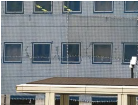
Photo 3.44 Damage of Tile on Exterior Wall
