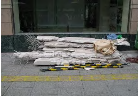
Photo 3.43 Dropped ALC Panels from 8 Story
