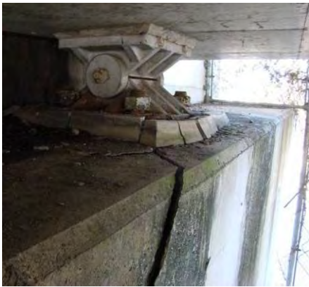
(c) Damage to Pier Top
