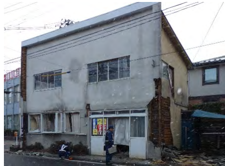
Photo 3.11 Drop Off the Mortar Wall (Komatsujima)
