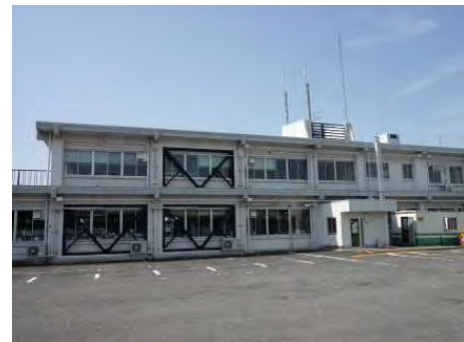
Photo 3.37 Appearance of Damaged Building
