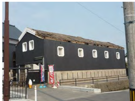
Photo 3.5 Warehouse with Mud Walls whose Roof System with Roof Tiles fell down
