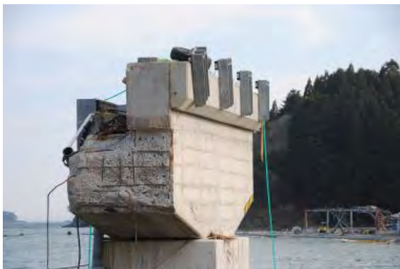
Photo 23 An upper steel bearing after damaged
