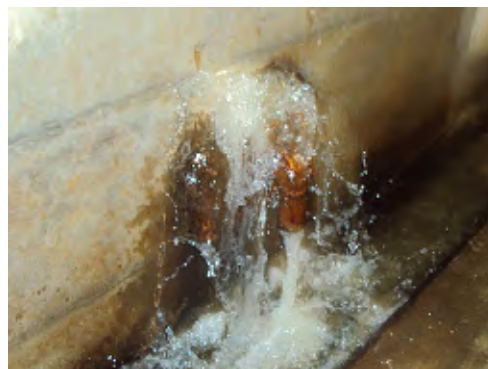
(b) Leakage from contraction joint 2J3
