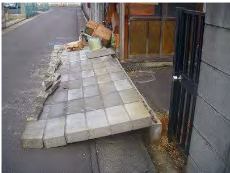
Photo 3.45 Collapse of Concrete Block Wall
