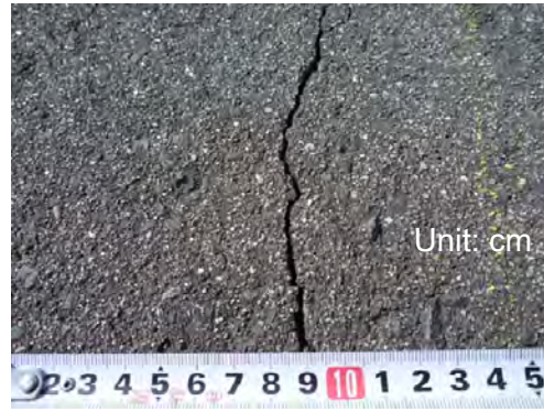
(b) Closeup of a crack
