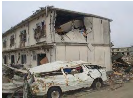
Photo 4.6 Wall Opening Generated by Debris Impact
