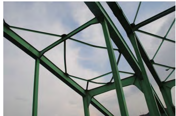
Photo 5 Buckled truss braces
