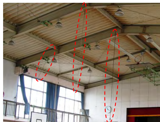
Photo 3.53 Fracture of Horizontal Brace
