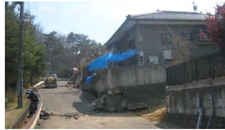
Photo 3.67 Damage of Retaining Wall and House Movement and Tilting by Sliding and Ground Transformation
