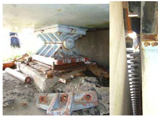
(d) Subsidence of Deck-End Resulting from Broken Movable Bearing
