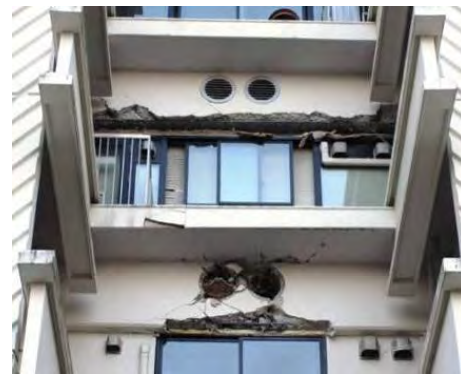
Photo 3.33 Damage on Boundary Beam with Opening
