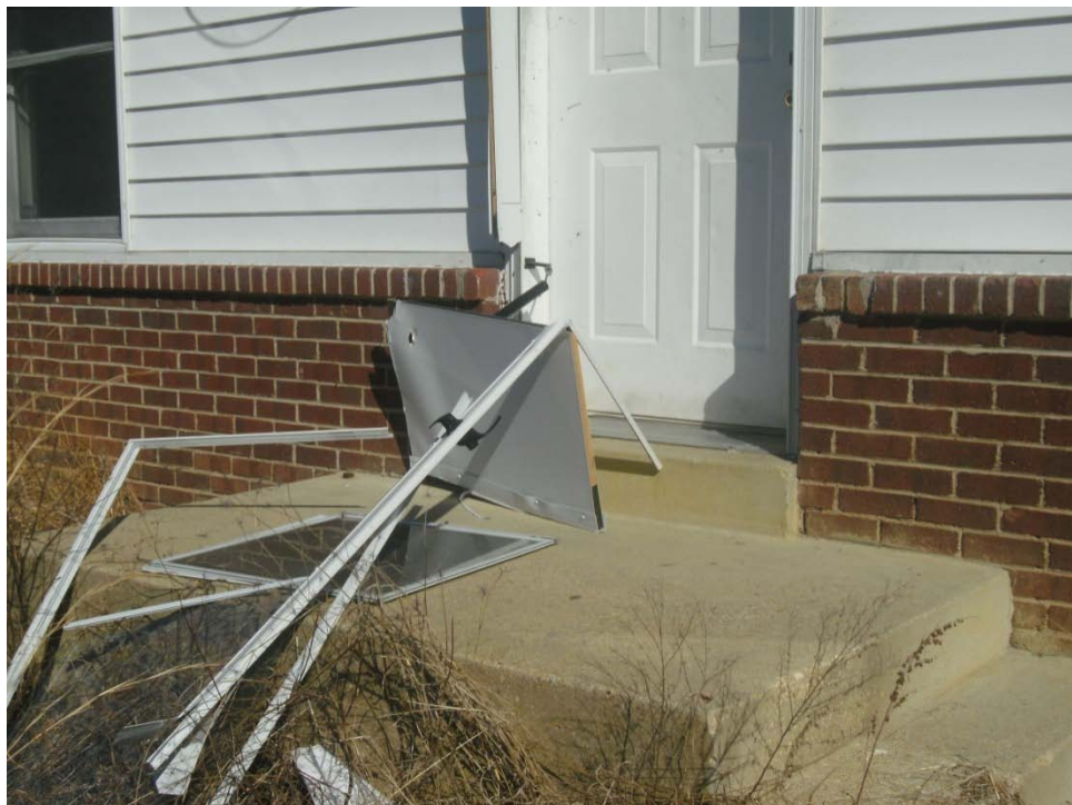
Debris from broken storm door at property 15204.
