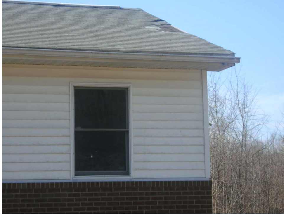
Damaged roof at property 15207.
