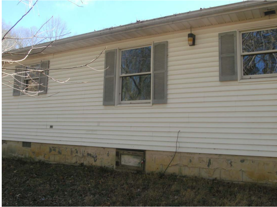
Foundation wall in need of repair at property 15200.
