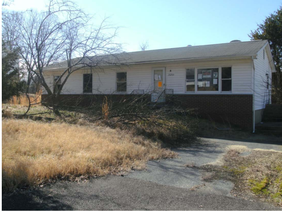
Fallen tree at property 15205. This property also had a broken window that is not visible in the picture.
