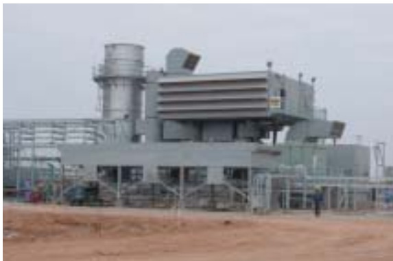
Iraq's first megawatt generator since 1976 is now operational. The 40-megawatt generator went online August 18, 2004 near Basrah, Iraq. Photo courtesy of U.S. Army.
