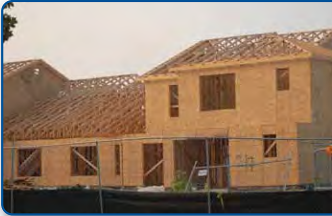
A junior-enlisted multiplex under construction at Dover Air Force Base. At project completion in 2009, the 212 homes constructed in 2004 - 2005 will be joined by 768 new homes.
