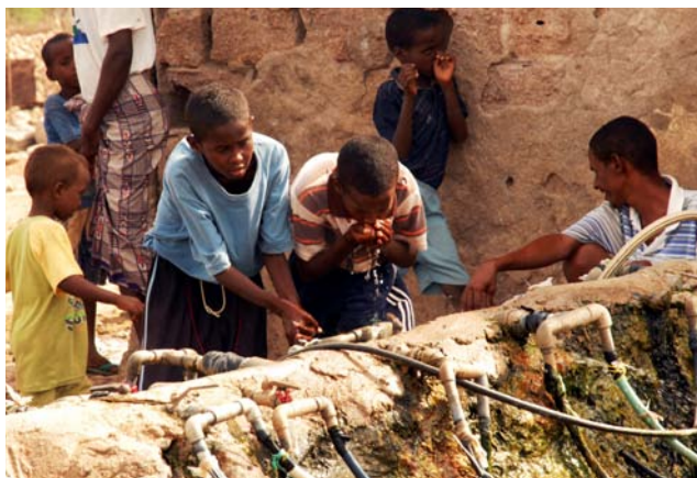
NAGAD, Djibouti — Children drink from the main water source in the village of Nagad, Djibouti on September 23, 2008. Seabees with Combined Joint Task Force - Horn of Africa (CJTF-HOA) were building a new water distribution system to separate drinking water from non-potable water. (Photo by U.S. Navy Petty Officer 2nd Class Ronald Gutridge)
