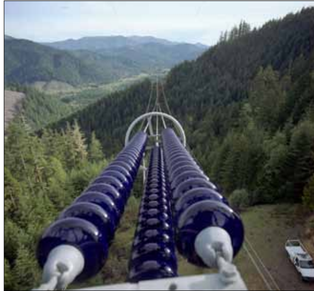
Birdseye view of insulators and transmission lines (photo courtesy Rocky Mountain Power Company and Idaho Power Company)
