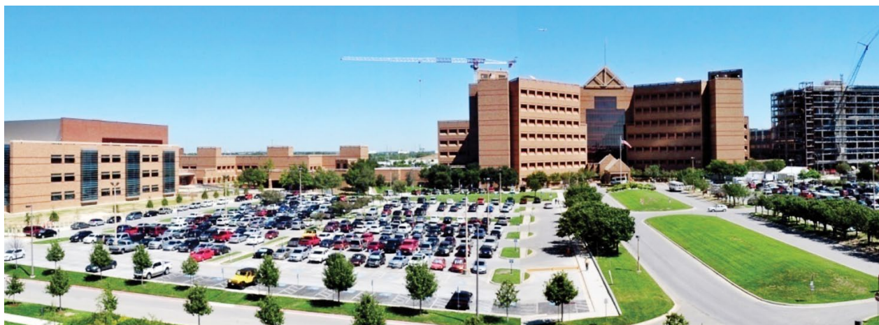
Construction continues on the new wing of the San Antonio Military Medical Center – North (formerly known as Brooke Army Medical Center), Fort Sam Houston, Texas.
