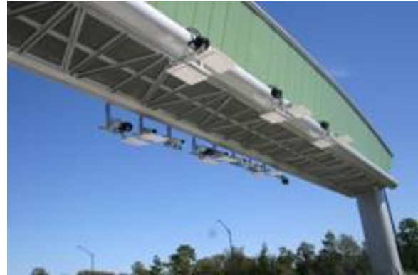
Figure 4-28. Florida Turnpike’s Overhead Gantry for ORT Allows for Maintenance Activities without Road Closure
