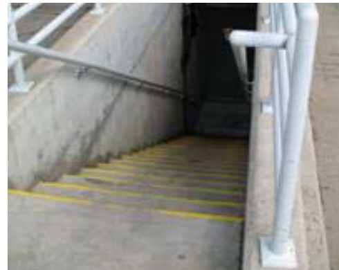
Figure 4-18. Handrails on Both Sides of Tunnel Stairways Can Improve Safety
