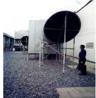
Terry Sharp, of ORNL, assesses energy savings opportunities at the Atlanta Federal Center.
