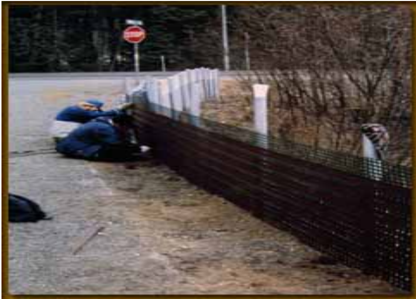
File dc-40: In areas along the stream where the riparian zone is very narrow or nonexistent, snow fences have been built to reduce the amount of snow and sand from entering the stream. Americorps volunteers have assisted in the installation and evaluation of these fences.
