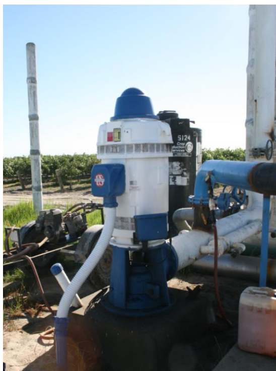
An irrigation pump connected to a web-to-wireless controller designed by M2M Communications.
