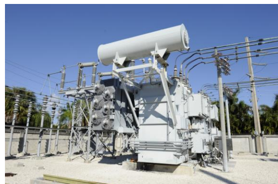
Smart devices have been installed on 78 substation transformer banks.
