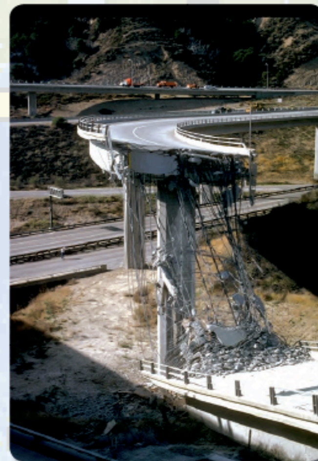
Collapse of the Interstate-5/State Highway-14 interchange showing damage north of Los Angeles caused by the 1994 magnitude 6.7 Northridge, California, earthquake. Thousands of State and County bridges were shaken at varying intensity levels during this earthquake; many required inspections.
