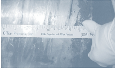
Measuring a crack discovered in a weld in a reactor coolant system pipe.
