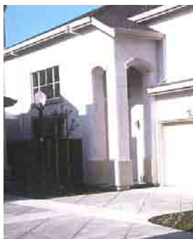
POORLY PROPORTIONED ENTRY COLUMN
