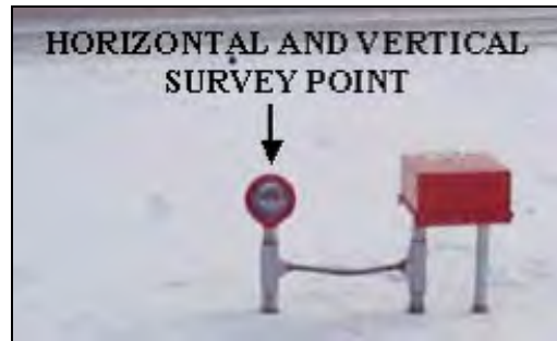
Figure C-4. Typical installation of the runway end identification light (REIL) with the horizontal and VSPs identified.
