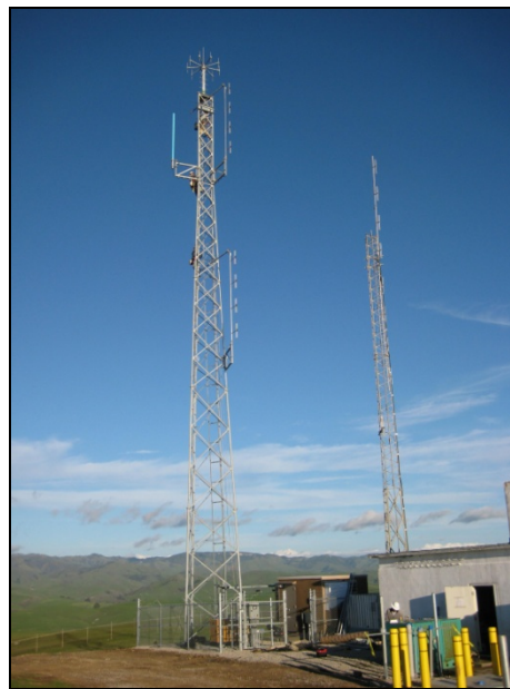
R21 tower in San Onofre, California (Permanent co-located infrastructure)
