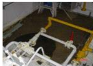
Fueling Piping System
