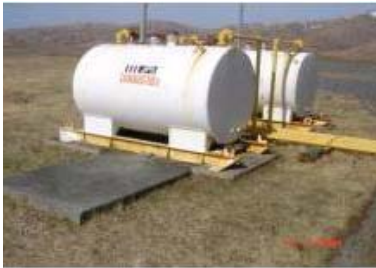
Exterior Fuel Tanks
