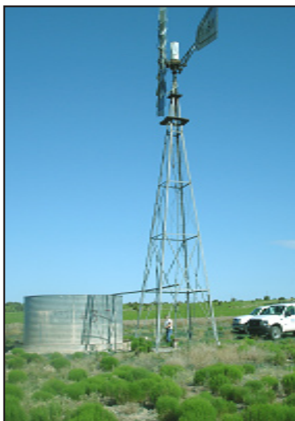
The Pueblo of San Felipe repaired and rehabilitated windmills, using NAAP funding.
