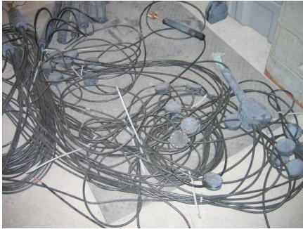
Figure 7: Fan wire antenna in a pile on the floor
