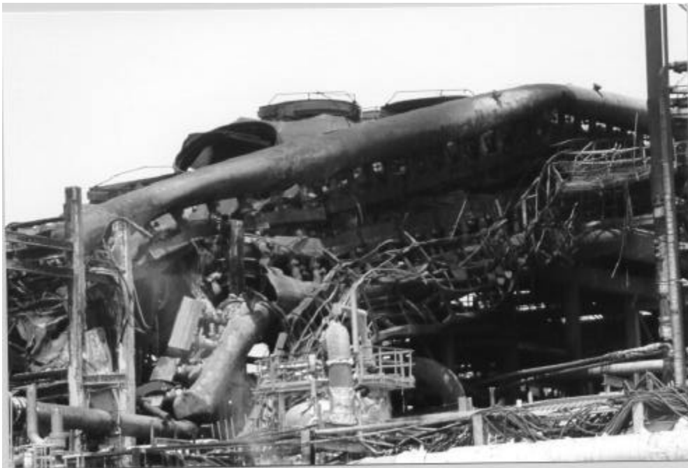
Figure E-2: Close-up of OP-III damage. The structure supporting the overhead cooling fans melted due to the intense heat of the fire and collapsed on top of the pipe rack.
