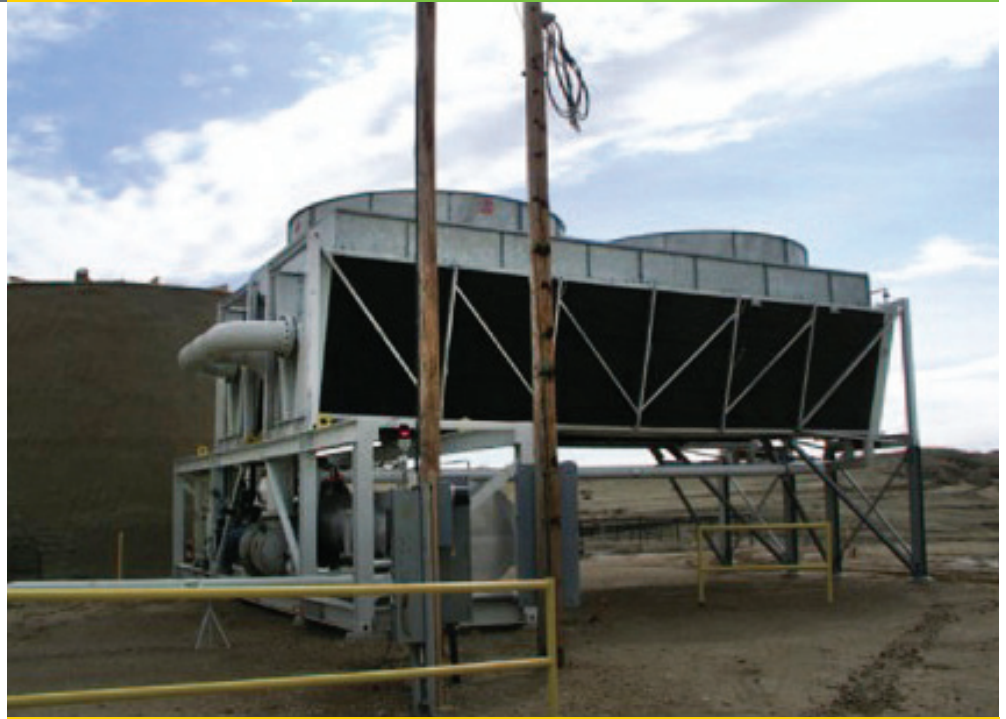
The Rocky Mountain Oilfield Testing Center in Wyoming was one of the first projects to validate the use of co-produced geothermal fluids from oil and gas wells for power generation. The binary cycle plant, shown here, produces approximately 200 kW of electricity.
