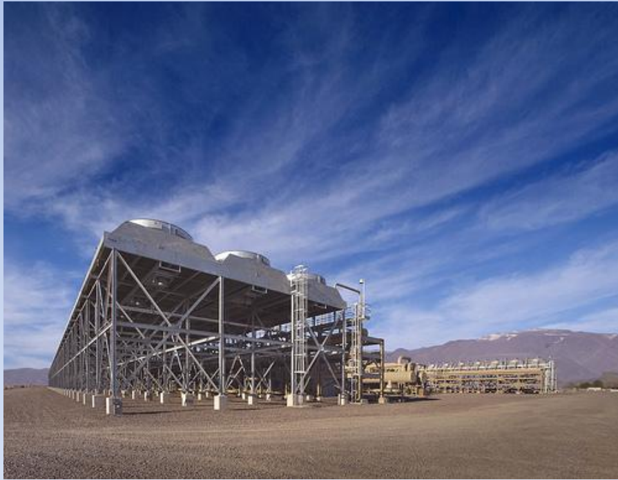
Stillwater Power Plant, NV
