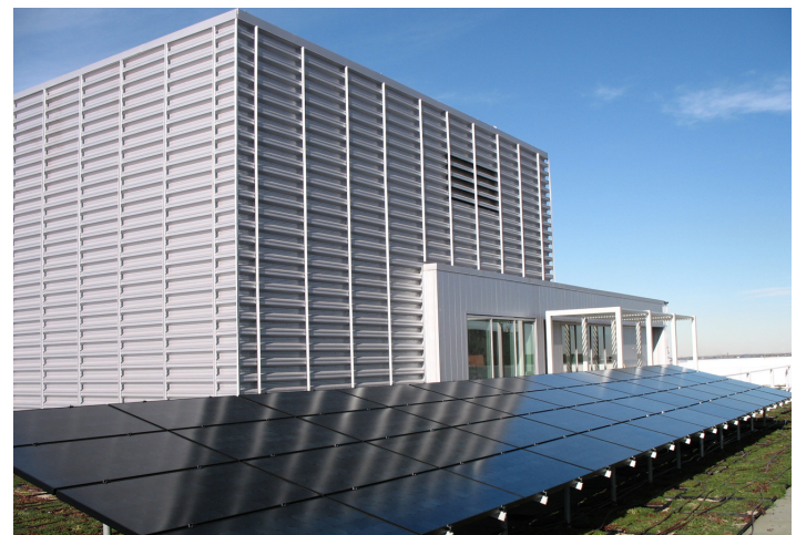
Forty-eight solar panels output 10kW at peak sun.
