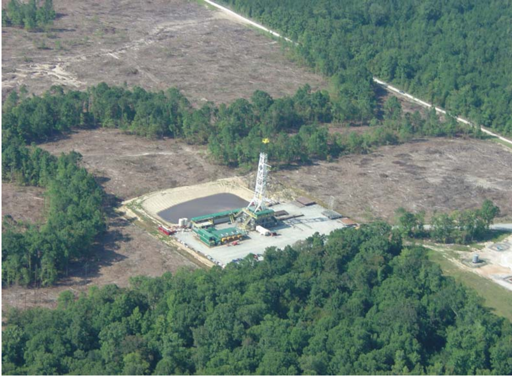
A Jackson Parish's well site
