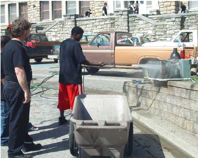
A faculty volunteer from the refrigeration and heating program at the Herndon Career Center in Lee's Summit, MO, shows volunteers how to clean air conditioning units at Westport High School in Kansas City, Mo.
