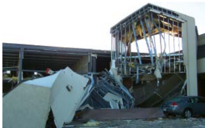
Prattville Station, Ala., was damaged during a recent tornado. Windows were broken at the station and damage occurred to one government vehicle.
