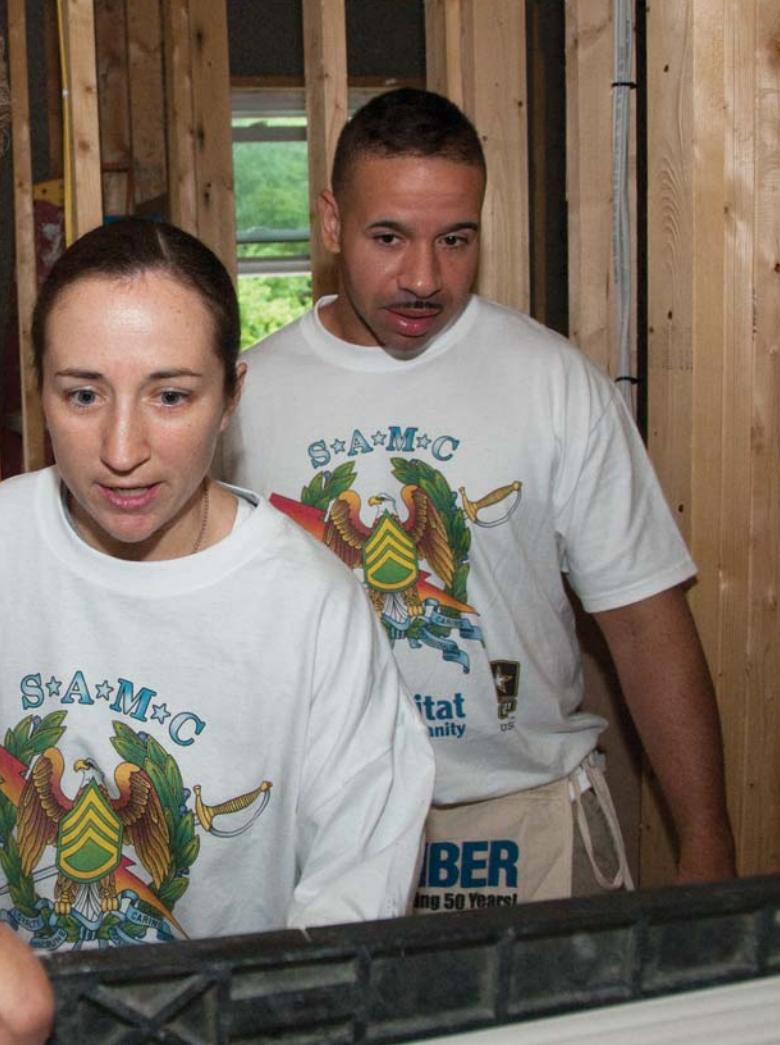
Bruce Singer, Hardin County Habitat for Humanity, helps Sgts. 1st Class Lindsay Dally and Ashford Harrison measure and cut drywall for installation at the Hardin County Habitat home build Aug. 4. Left: Sgt. 1st Class Carol Balderas installs a sheet of drywall. Top Right: Habitat construction foreman Howard Gatlin and Staff Sgt. Michael Schultz cut drywall for the ceiling.
