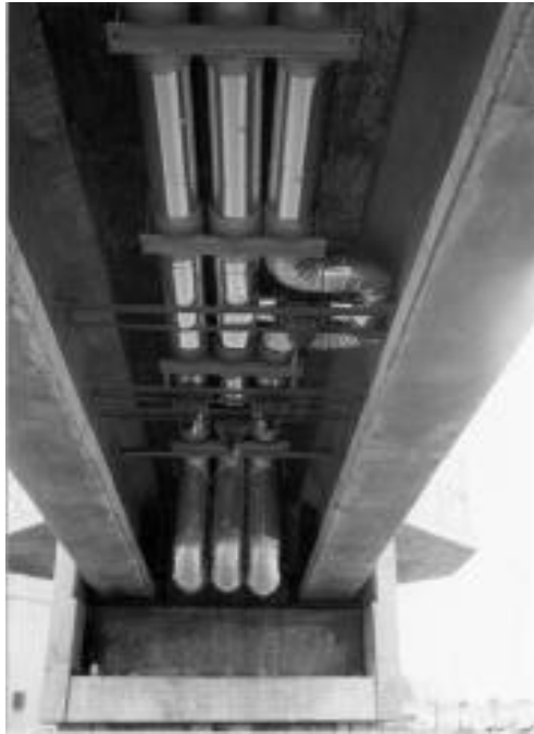
Fig. 2. Flexible expansion loops in supply/return pipes underneath walkway. View looking up.
