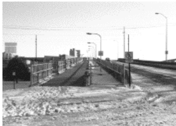
Fig. 7. Deck condition at hour 31.
