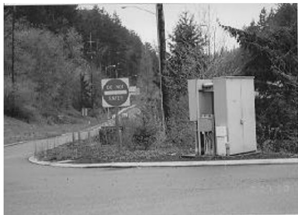
Fig. 4. South approach road looking east, heating control cabinet at right.
