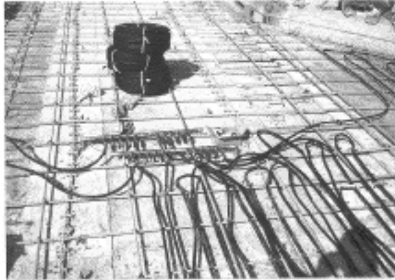
Fig. 3. Distribution manifolds are horizontal copper pipes in center which supply the rubber hydronic tubes.
