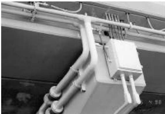
Fig. 3. Close-up of supply and return manifolds (pipes in center) and thermocouple conduits terminating in enclosure at right.
