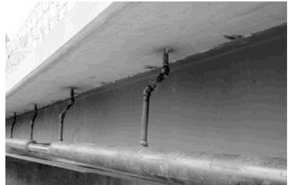
Fig. 5. Risers deliver heated working fluid to a series of evaporators, each serving 10 Perkins tubes in bridge deck.
