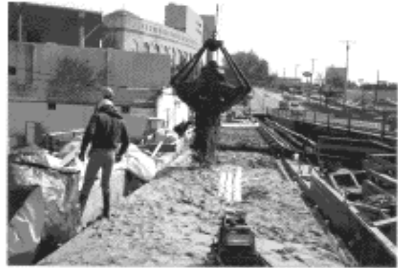
Fig. 4. Uninsulated PVC supply and return pipes were bedded in sand in approaches on both ends of walkway.
