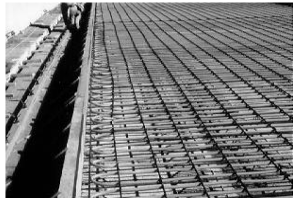
Fig. 4. Heating hoses in place ready for concrete pour; hoses are on 152 mm (6-in.) centers placed 76 mm (3 in) under top of slab, affixed below #4 rebars.
