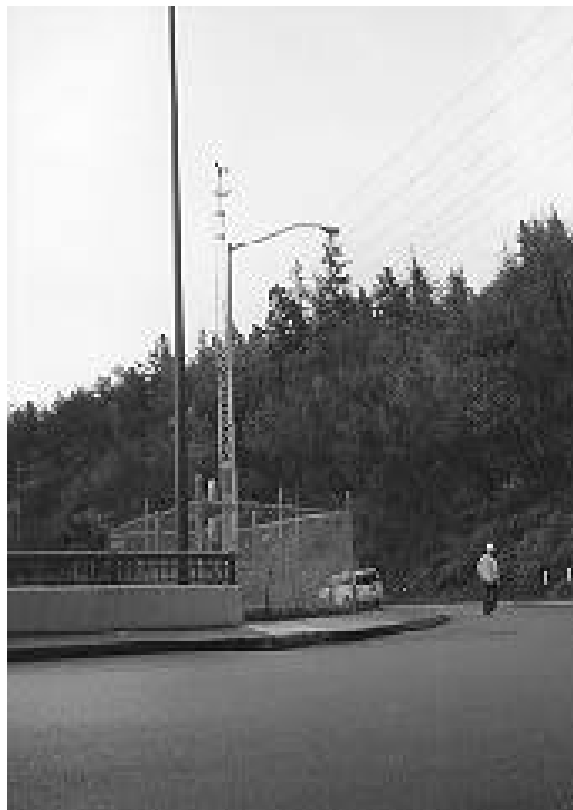
Fig. 5. Met station is located at south end of heated deck, opposite control cabinet.
