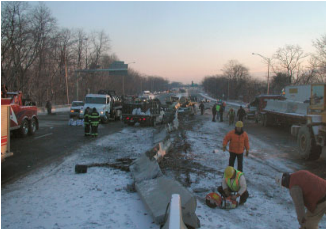
Figure 10. Overturned portable concrete barrier segments viewed from northbound lanes of I-95.
