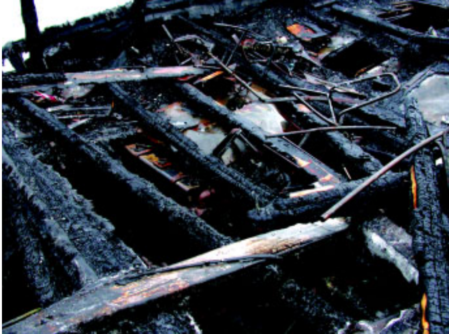
Figure 9. Debris over the engine compartment that investigators had to remove before they could examine the Express Shuttle II 's engines and generators.
