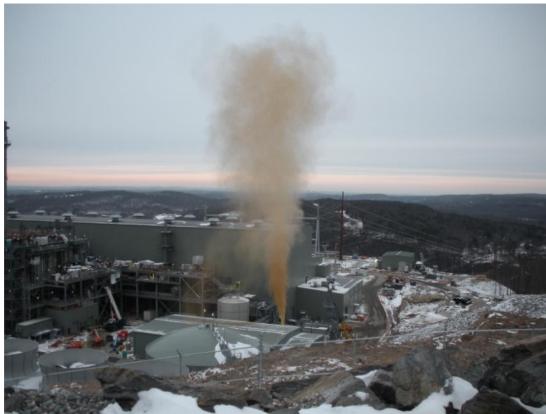
Figure 3. The cleaning of fuel gas piping at the Kleen Energy site on January 30, 2010, one week prior to the incident; a “gas blow” method was used to remove debris from the piping. The brown cloud seen here is indicative of debris being blown from the line.
