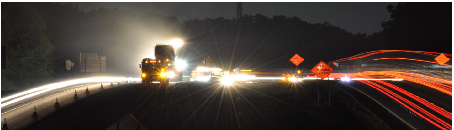
TDOT crews work to resurface a section of Interstate 24 in Coffee County, Tennessee, under cover of darkness. Photo courtesy of Tennessee Department of Transportation.
