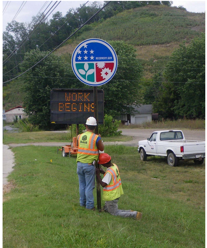
TDOT crew installs Recovery Act logo signage along state Route 66 in Sevier County, Tennessee. Photo courtesy of Tennessee Department of Transportation
